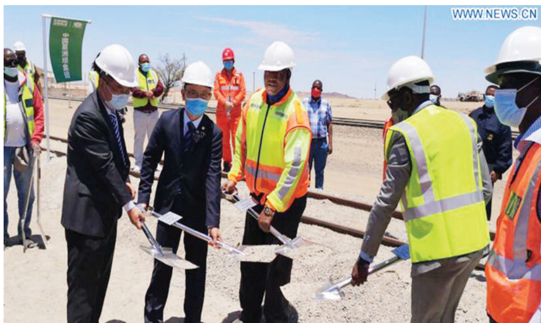
Officials from Namibia's Ministry of Works and Transport and China's Gezhouba Group Corporation in Namibia break ground for the rehabilitation and upgrading of the railway between Walvis Bay and Arandis in Arandis, western Namibia, on Nov. 30, 2020.
