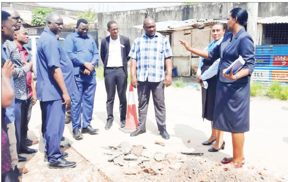
Lydia Ndebalema (R), a director with the Dar es Salaam Water and Sanitation Authority, briefs Kinondoni district commissioner Daniel Chongolo (3rd-R) yesterday at the site where the agency is implementing a sewage system project to serve Mwananyamala referral hospital's maternity ward. Photo: Guardian Correspondent
