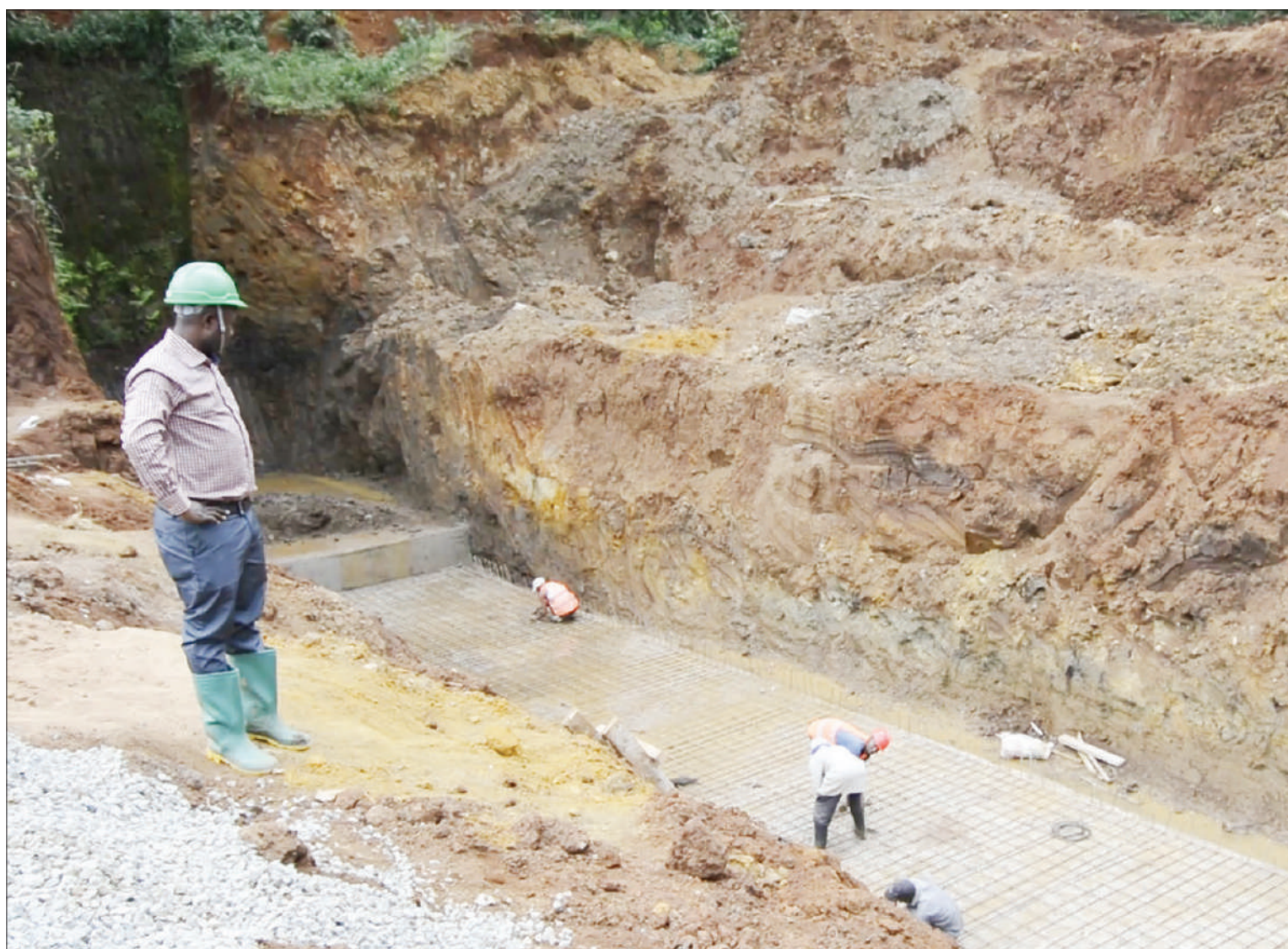
Kilimanjaro regional irrigation engineer Saidi Hussein has an eyewitness account of the ongoing construction of a wall around Orumwi Dam at Kishisha in Siha District on Thursday. The project is being implemented in line with one of former president Dr John Magufuli's 2020 General Election campaign pledges. Photo: Correspondent Mary Moshia
