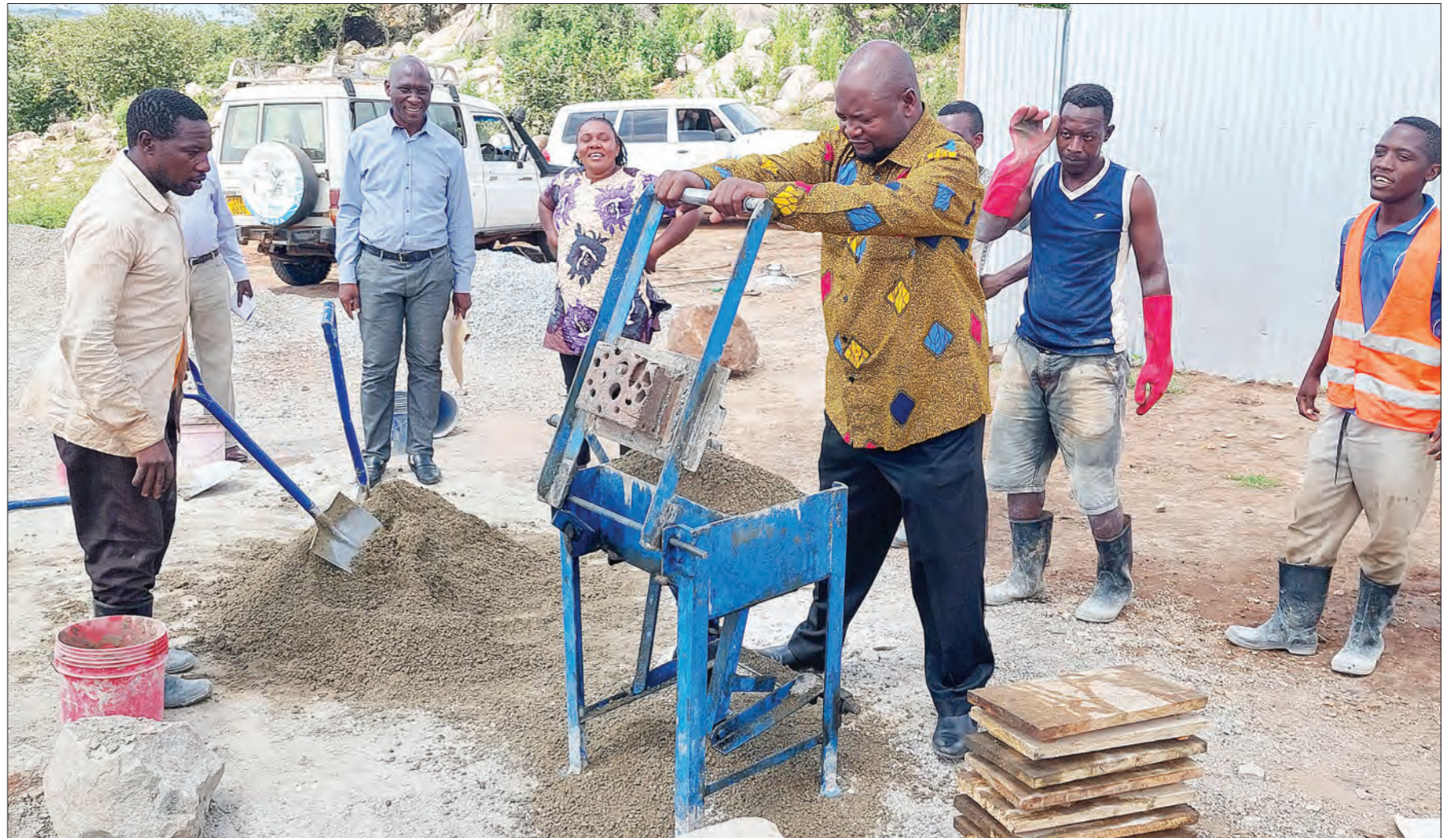
Kahama district commissioner Festo Kiswaga lends a hand in the making of bricks for the construction of a 1,000-litre water tank at Itumbili village in Chambo ward earlier this week. He was on an inspection tour of the implementation of development projects. Photo: Correspondent Shaban Njia.
