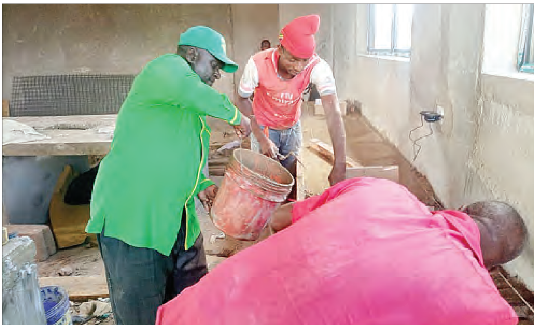
Yohana Maitei Kadogoo (L), councillor for Ruvu Remit ward in Simanjiro District, joins technicians in the construction of a laboratory at Ruvu Remit Secondary School on Thursday. Photo: Correspondent Gift Thadey
