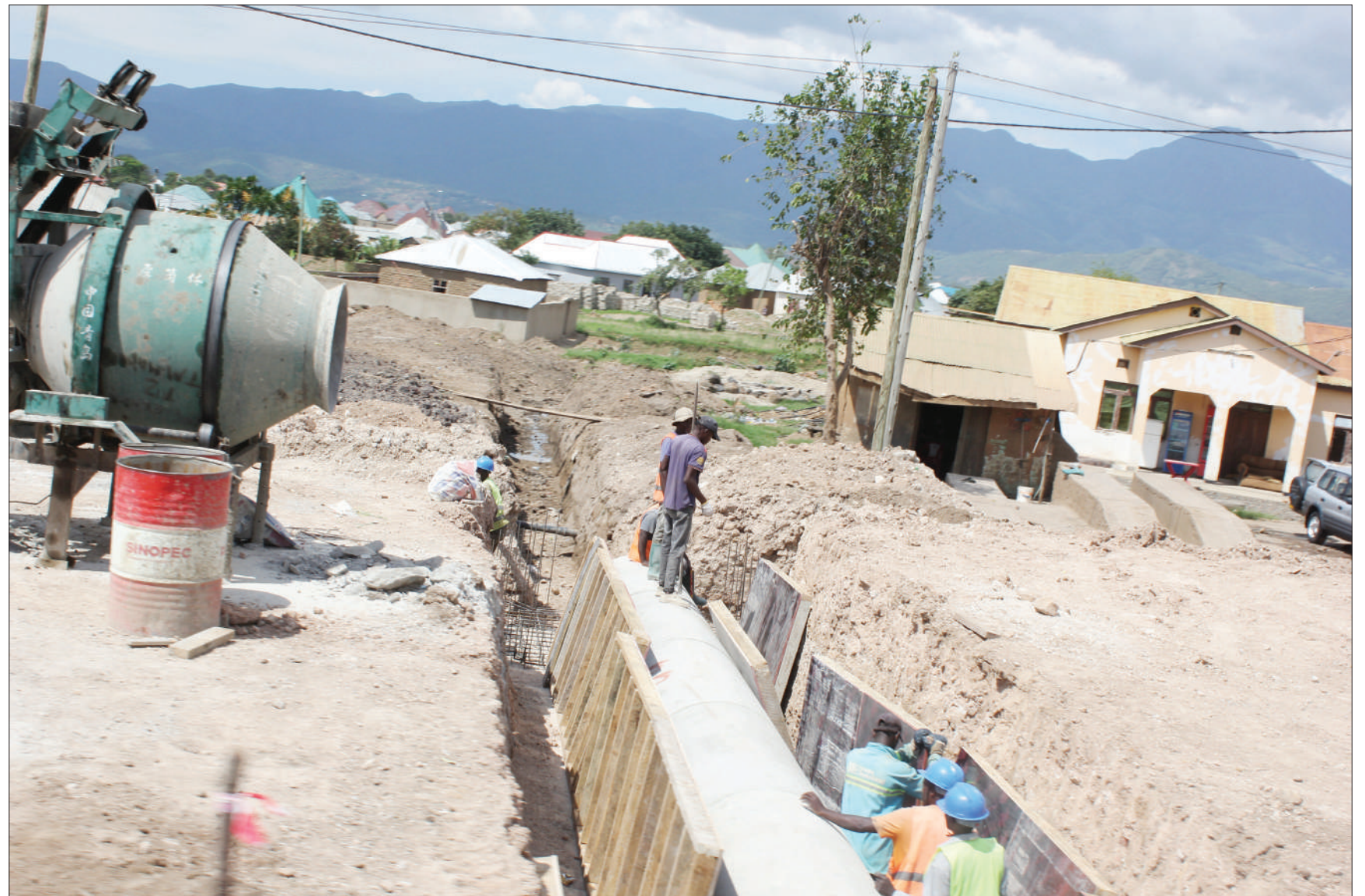
Construction of sewage system in progress yesterday at Mwakapangala in Mbalizi town along the 29-km four-lane section of road being built from Nsalaga in Mbeya city to Songwe International Airport. Photo: Correspondent Nebart Msokwa
