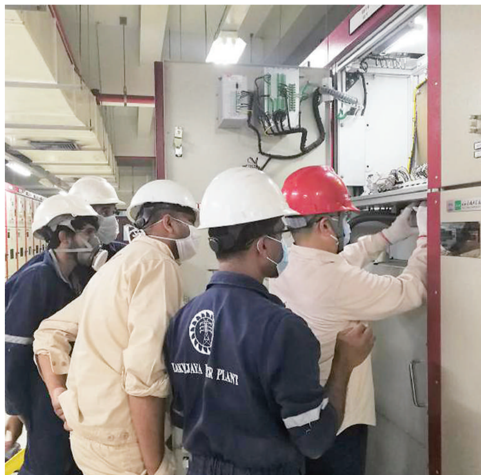
Chinese and Sri Lankan staff members conduct maintenance work at Lakvijaya Power Station in Puttalam, Sri Lanka, April 11, 2020. Photo: Xinhua
