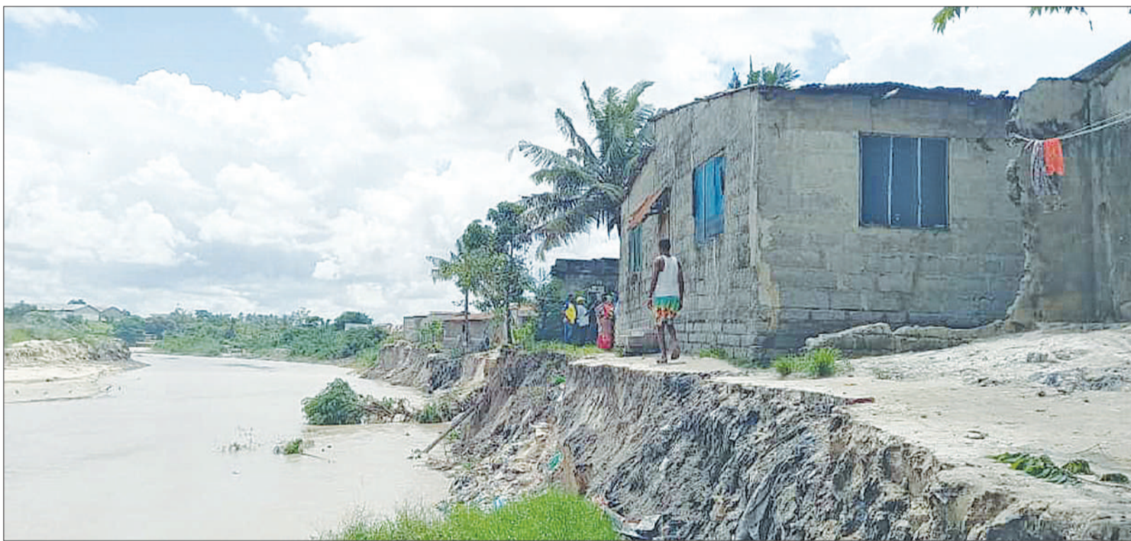
This is but one of several houses in Dar es Salaam's Tabata Liwiti suburb risking imminent collapse should raging floodwaters continue to eat away the banks of this section of the Msimbazi River just inches away. Correspondent Pilly Kigome captured this scene yesterday.
