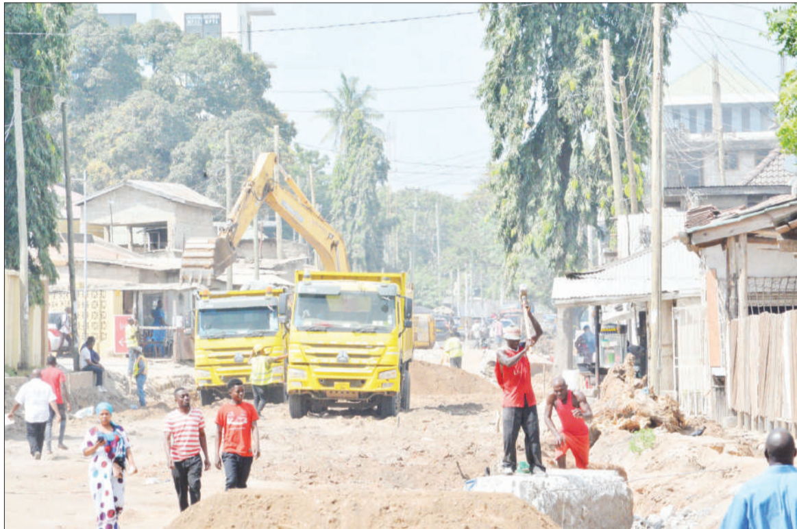
Improvement of roads in Kinondoni District, Dar es Salaam, well under way - as found yesterday. Photo: Correspondent Miraji Msala
