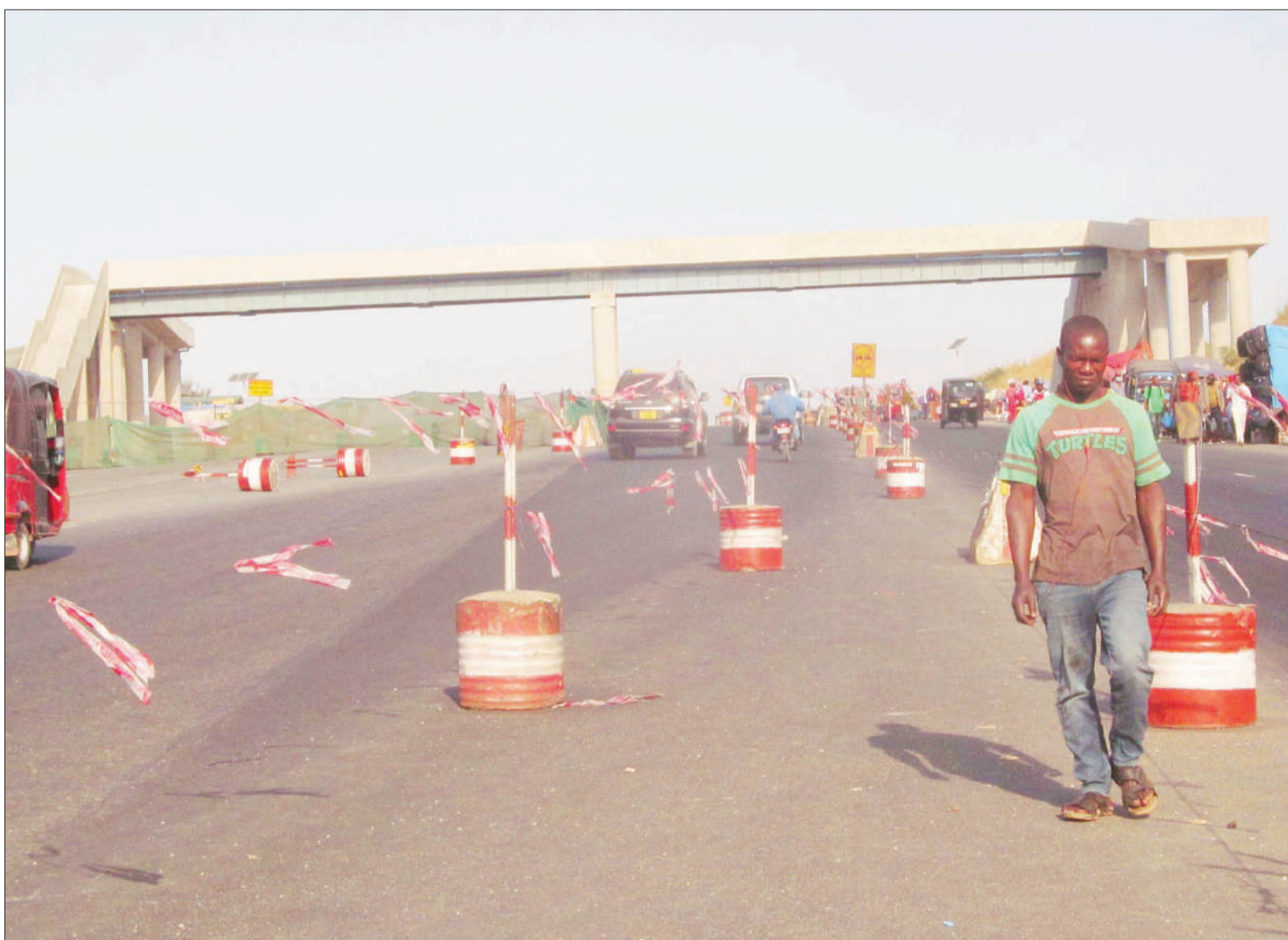
Construction of a pedestrian flyover at a Mbezi Mwisho section of Dar es Salaam's Morogoro Road as good as complete, as witnessed yesterday. Photo: Correspondent Sabato Kasika
