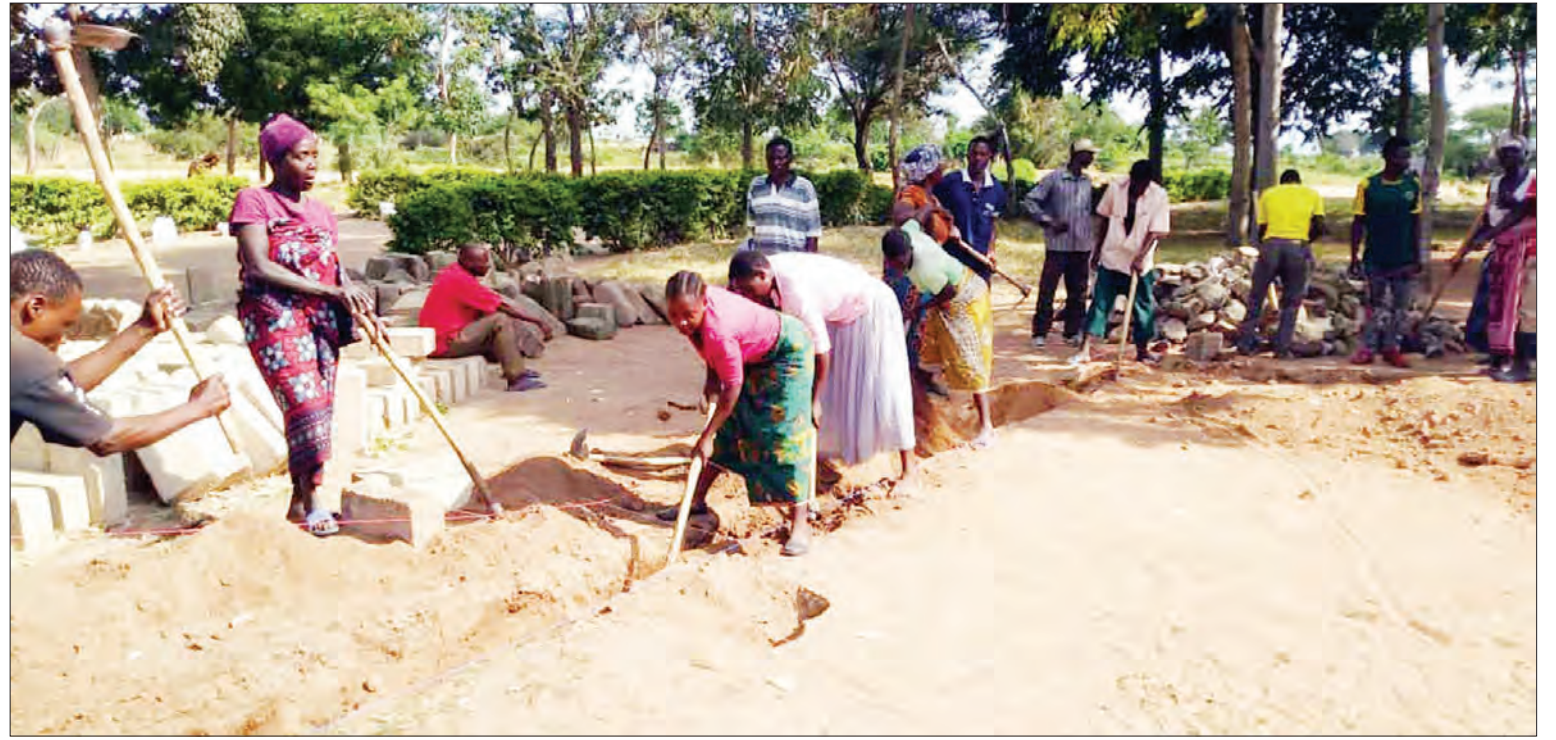
Residents of Mugango ward in Musoma District participate in the digging of the foundation for the library building at Karubugu Primary School, as captured at the weekend. Photo: Guardian Correspondent
