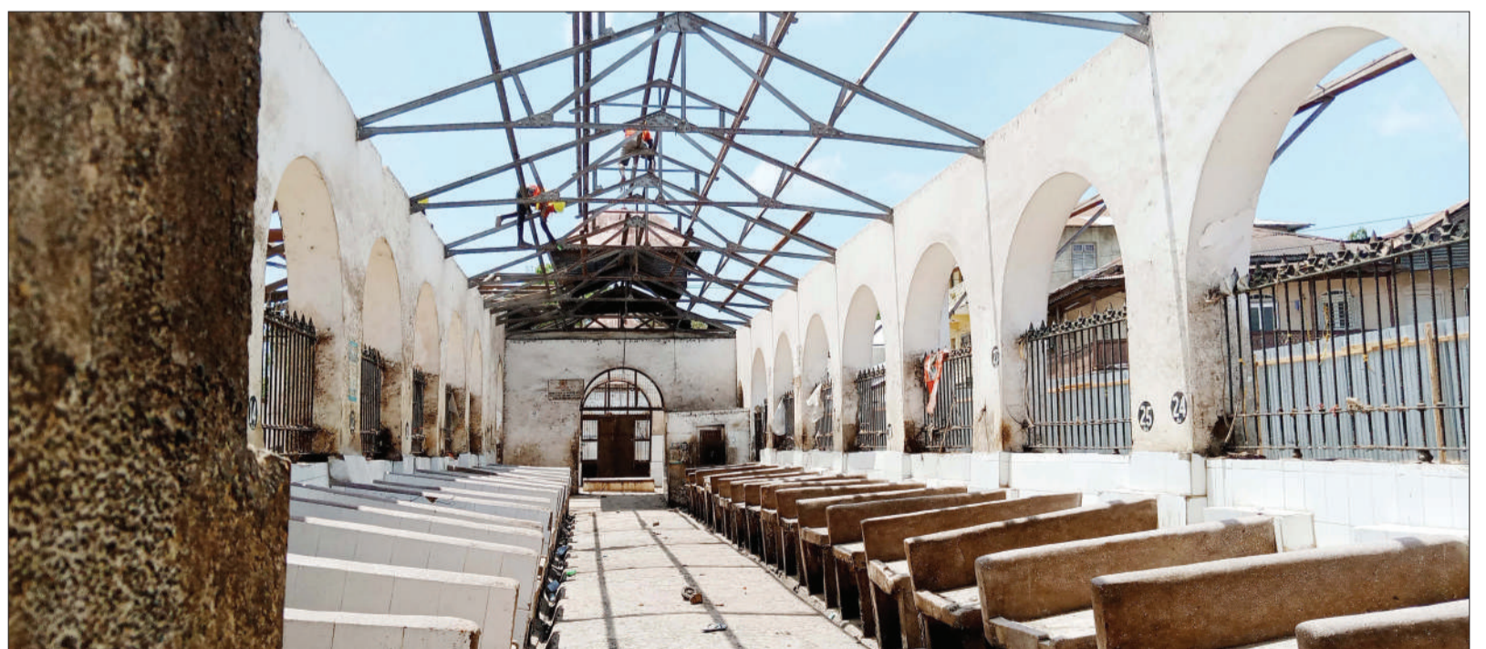
Rehabilitation of Zanzibar's 118-year-old Darajani main mixed-goods market in progress, as found yesterday. Photo: Rahma Suleiman
