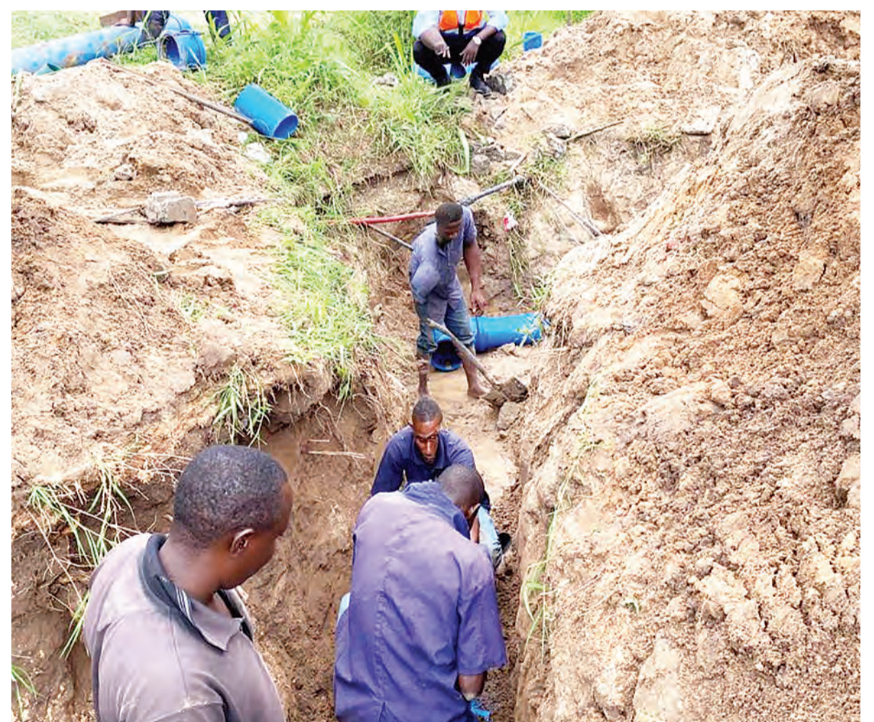
Dar es Salaam Water and Sanitation Authority (Dawasa) technicians move to repair a damaged pipe at Ulongoni B (Songsas) in Ilala District at the weekend. Photo: Correspondent Joseph Mwendapole
