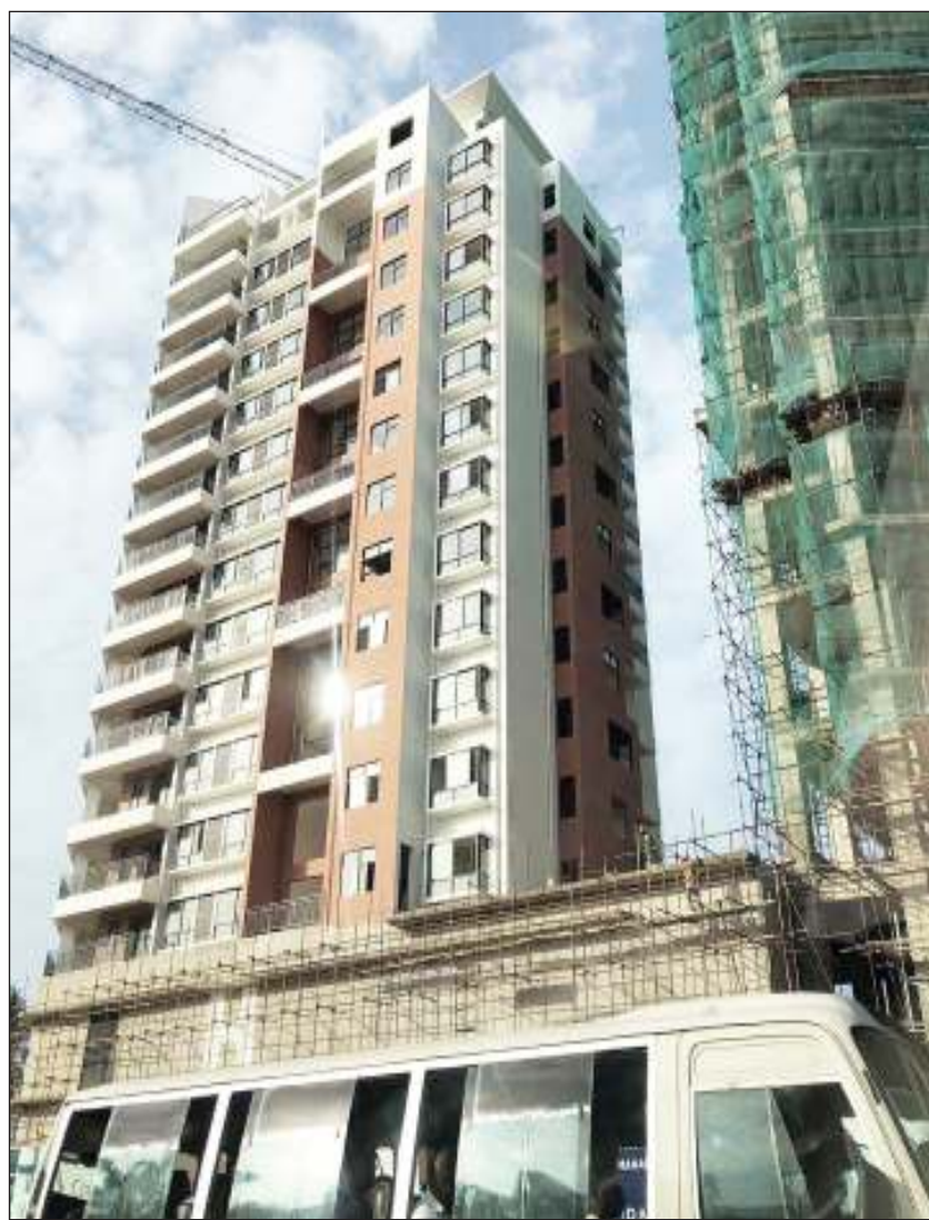
Construction work going on at Palm Village in Dar es Salaam, which will also have a 180-room hotel. Photo courtesy of Ivory Towers Limited.
