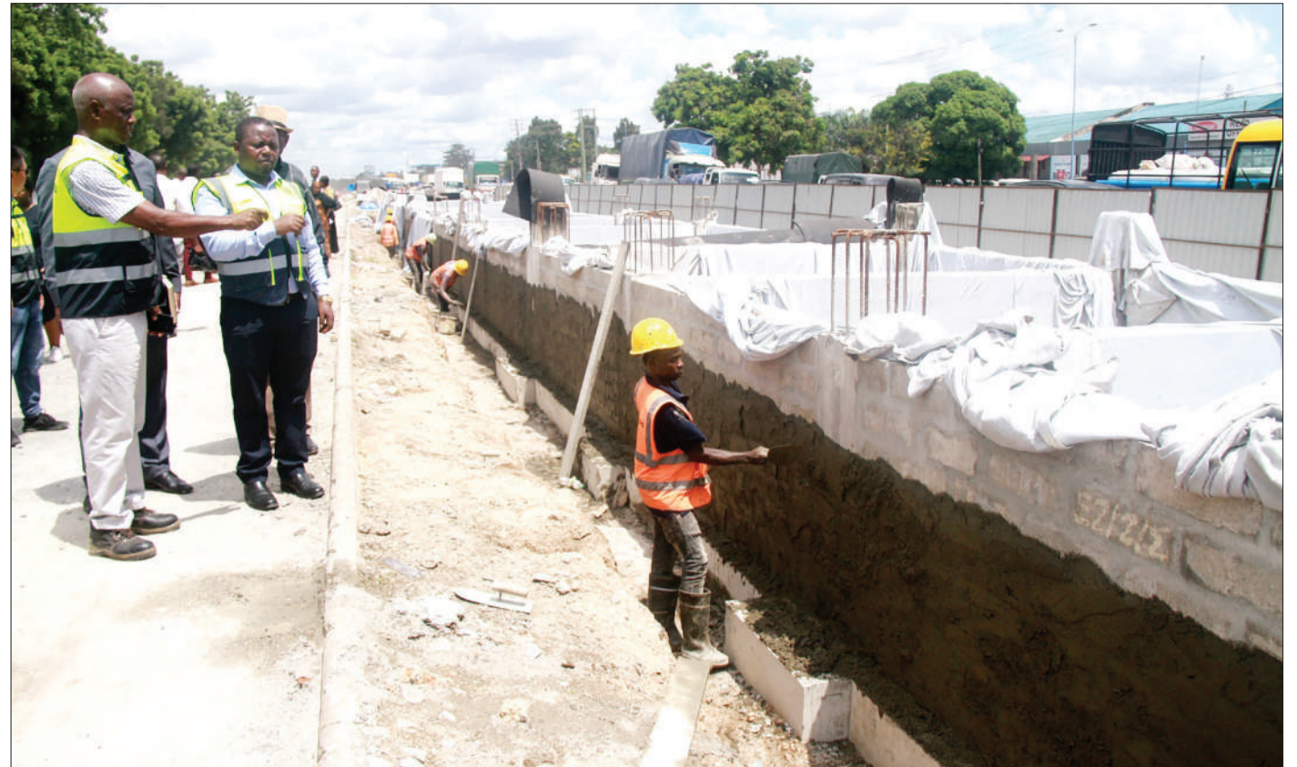
Barakaeli Mmari (L), a manager with Dar es Salaam's Bus Rapid Transit project, briefs Tanzania National Roads Agency (Tanroads) CEO Rogatus Mativilia (2nd-L) yesterday as the latter made an assessment tour of progress on the Gerezani-Gongo la Mboto stretch. Photo: Correspondent Jumanne Juma
