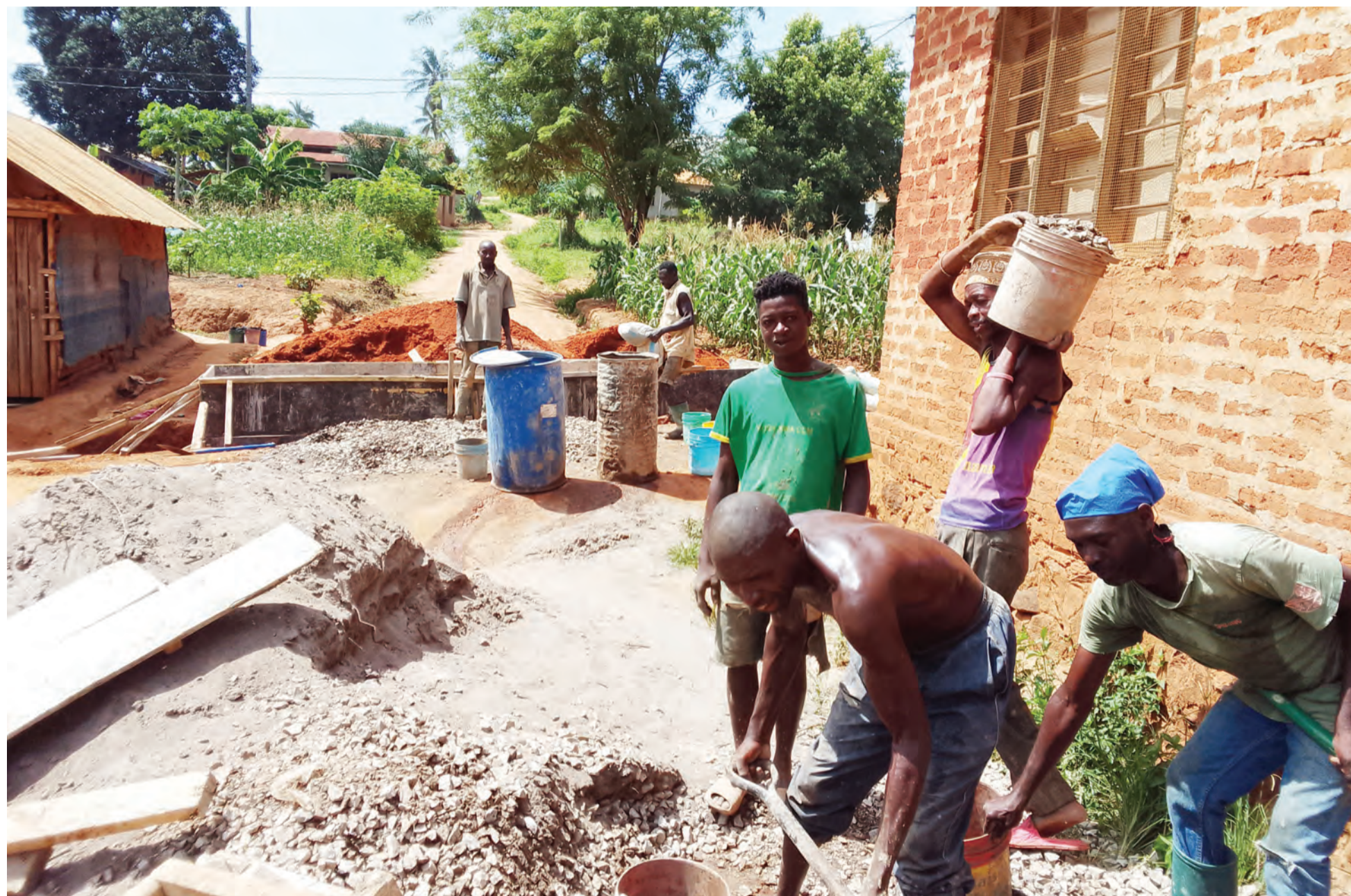
Workers in progress of the culvert bridge construction on the road leading to the Kwamkabara Ward Executive Office in Muheza District, Tanga Region, recently. Photo: Correspondent Steven William
