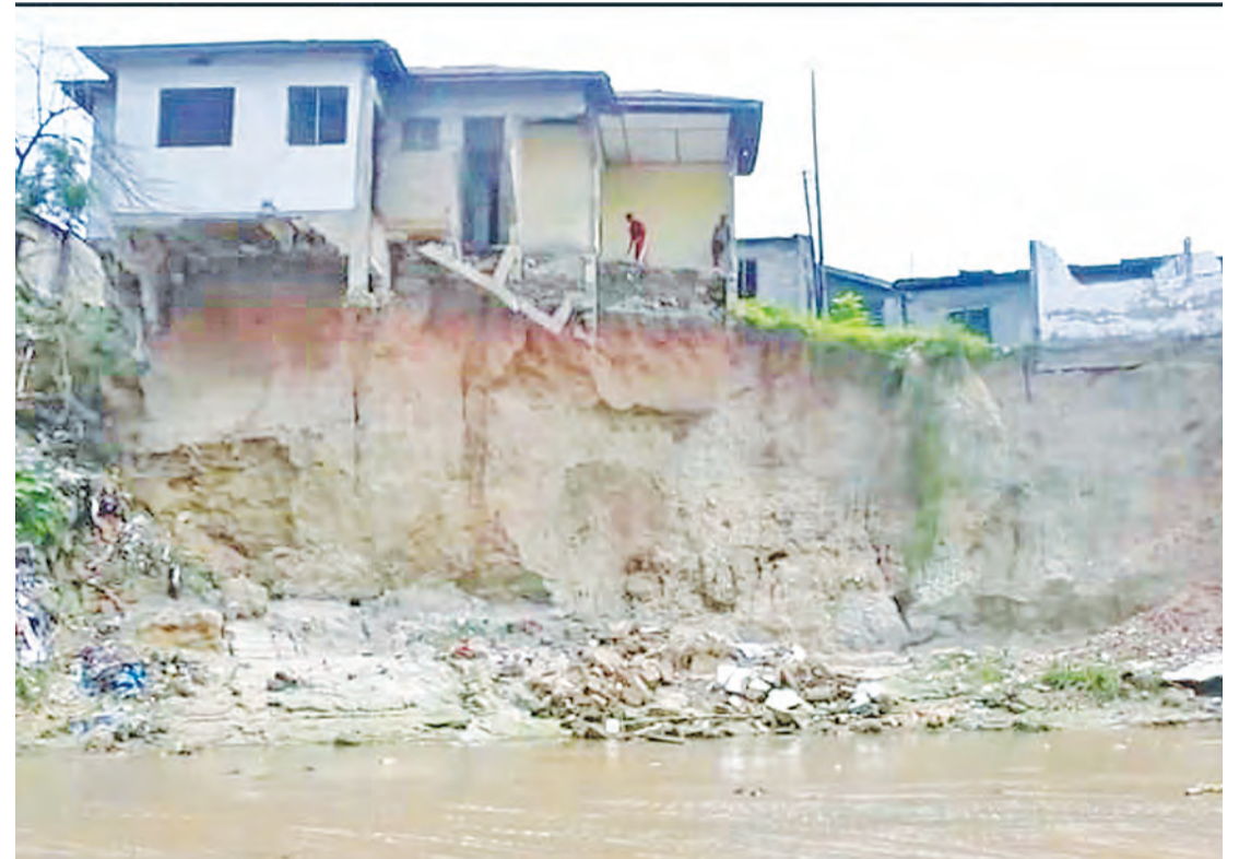
Residential houses along the Tegeta River were washed out by rainwater. Photo: Francis Kajubi
