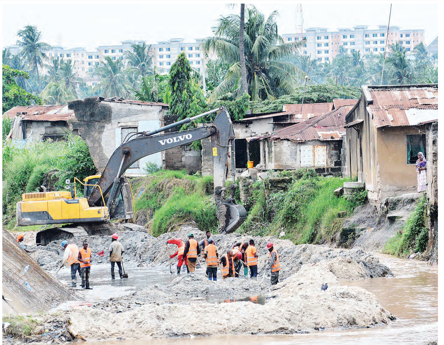
Preparations in progress yesterday for the construction of a concrete wall meant to prevent erosion by River Ng'ombe waters from further threatening surrounding areas in Dar es Salaam's Tandale suburb with collapse. Photo: Correspondent Miraji Msala
