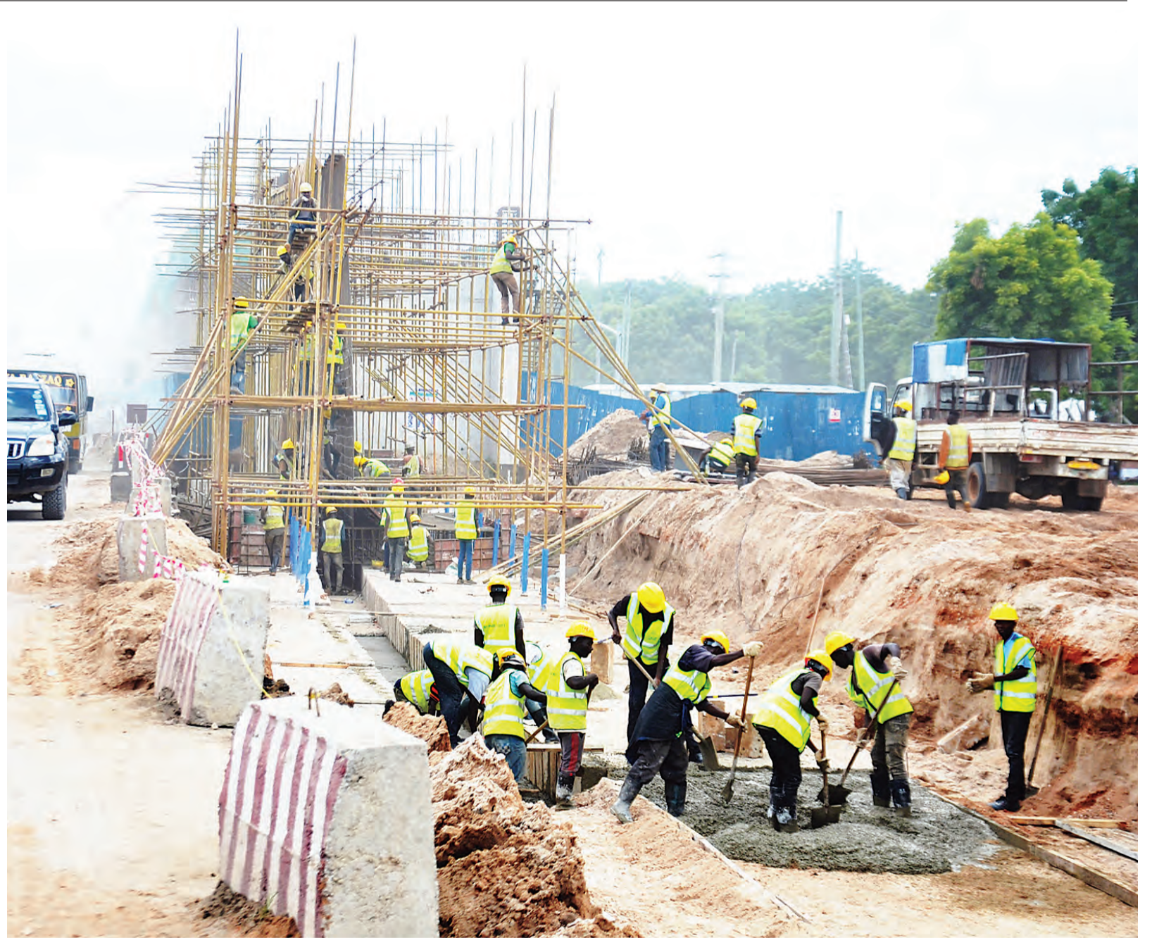
Construction of Uhasibu flyover at the Kilwa Road/Mandela Road junction in Dar es Salaam well under way, as captured yesterday. Photo: Correspondent Jumanne Juma
