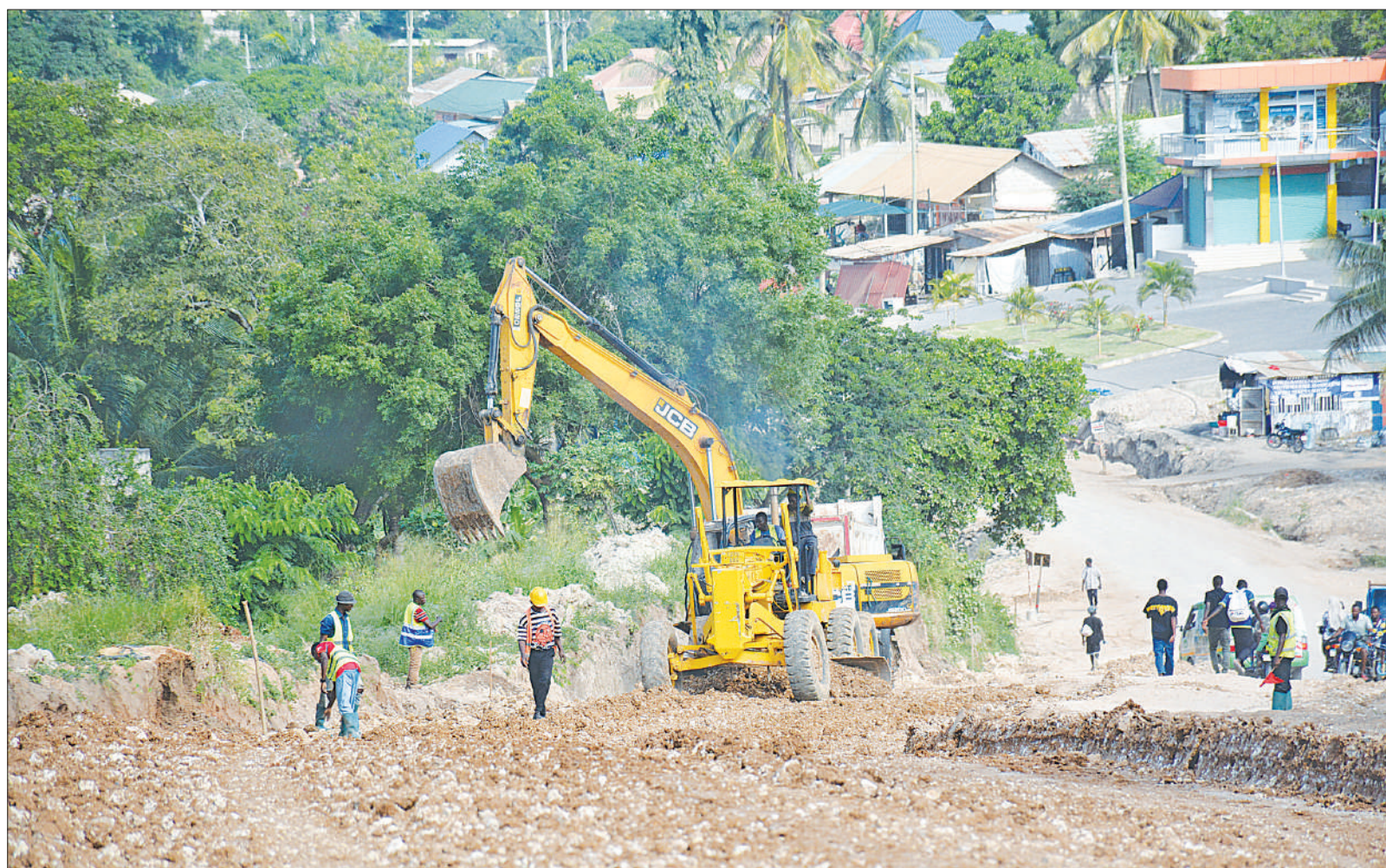
Construction of a road in Dar es Salaam's Matosa suburb (Ubungu municipality) to tarmac level in progress, as found earlier this week. Photo: Correspondent Miraji Msala
