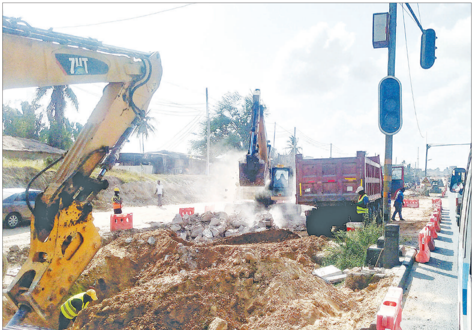
Workers continue with expansion of Morogoro Road at Kimara Bucha area in Dar es Salaam yesterday by converting it into a six-lane highway. Photo: Correspondent Sabato Kasika
