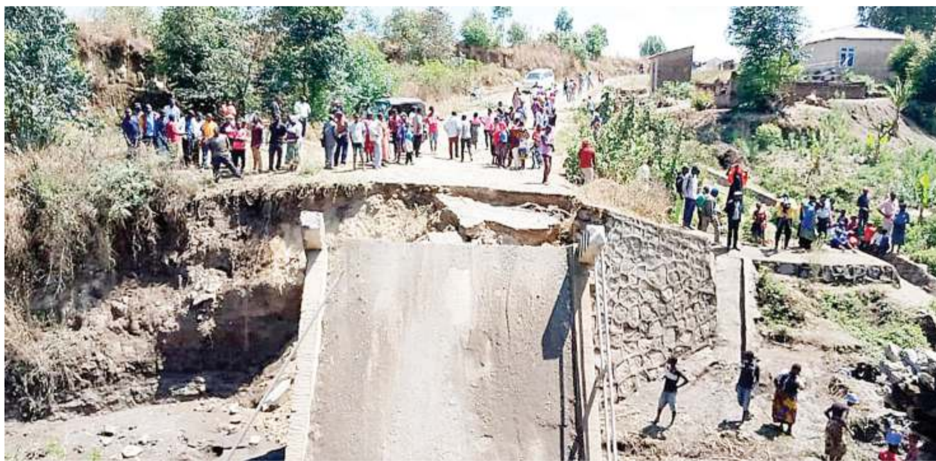
Mbeya city residents look on forlornly at the bridge supposed to connect Mbeya Region's Mwasanga and Mwakibete wards but now rendered impassable following destruction caused by ongoing rains. Photo: Correspondent Nebart Msokwa
