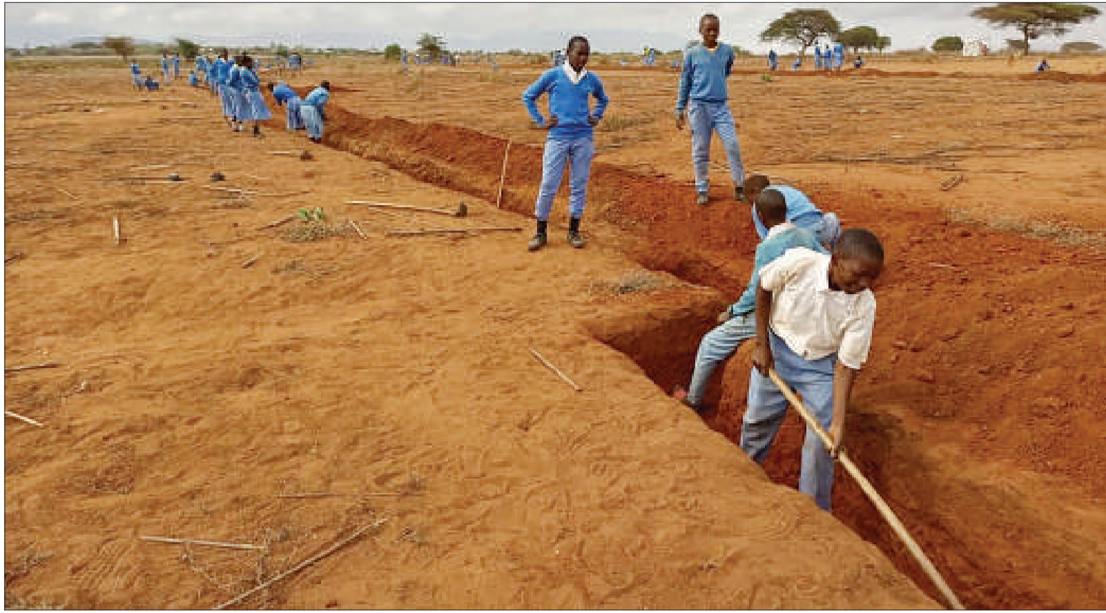
Students from Moletii secondary school in Kongwa district, Dodoma region erecting terraces on farms to improve water availability for plants and prevent soil erosion. Photo: Guardian Correspondent Valentine Oloro.
