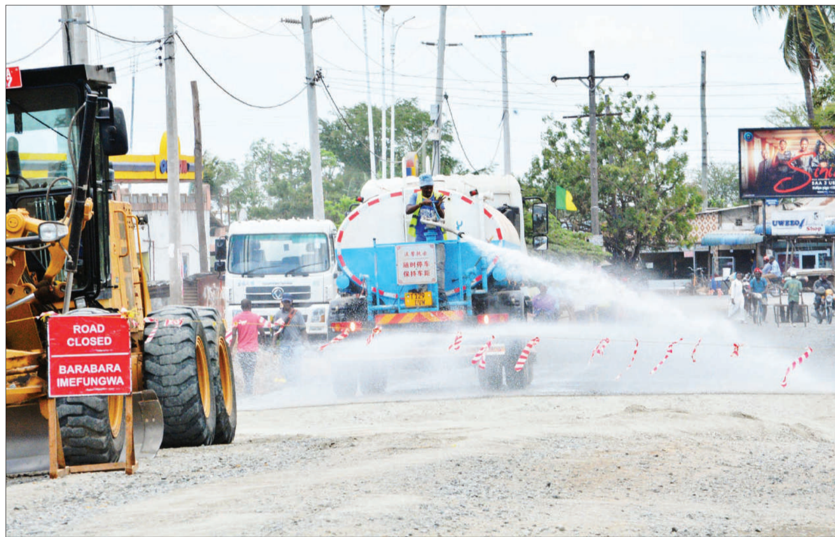
Construction of Mabibo road in the outskirts of Dar es Salaam progressing well as captured by our photographer yesterday. Photo: Correspondent Miraji Msala
