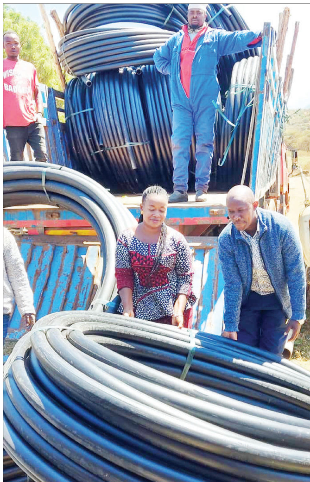
Hanang' district commissioner in Manyara region Janeth Mayanja (L) and Hanang' legislator Eng Samwel Hayuma inspect the consignment of water pipes being unloaded for distribution in Katesh township on Thursday. Photo: Correspondent Gift Thadey
