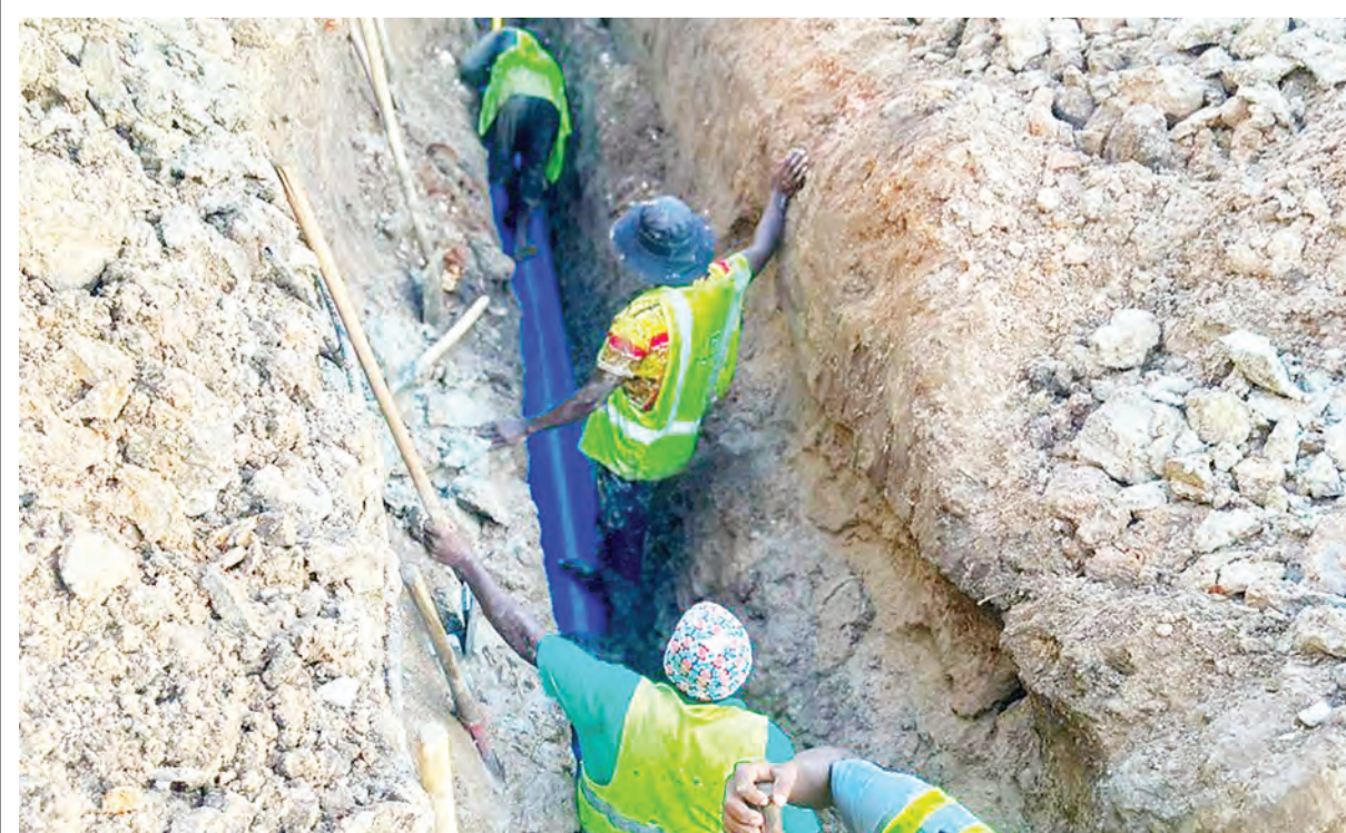
Technicians lay pipes for PSSF Sinza Kijitonyama sanitation project that will serve more than 1,000 residents of Sinza B, Sinza C Mabatini and Mananayama. Photo Correspondent Joseph Mwendapole
