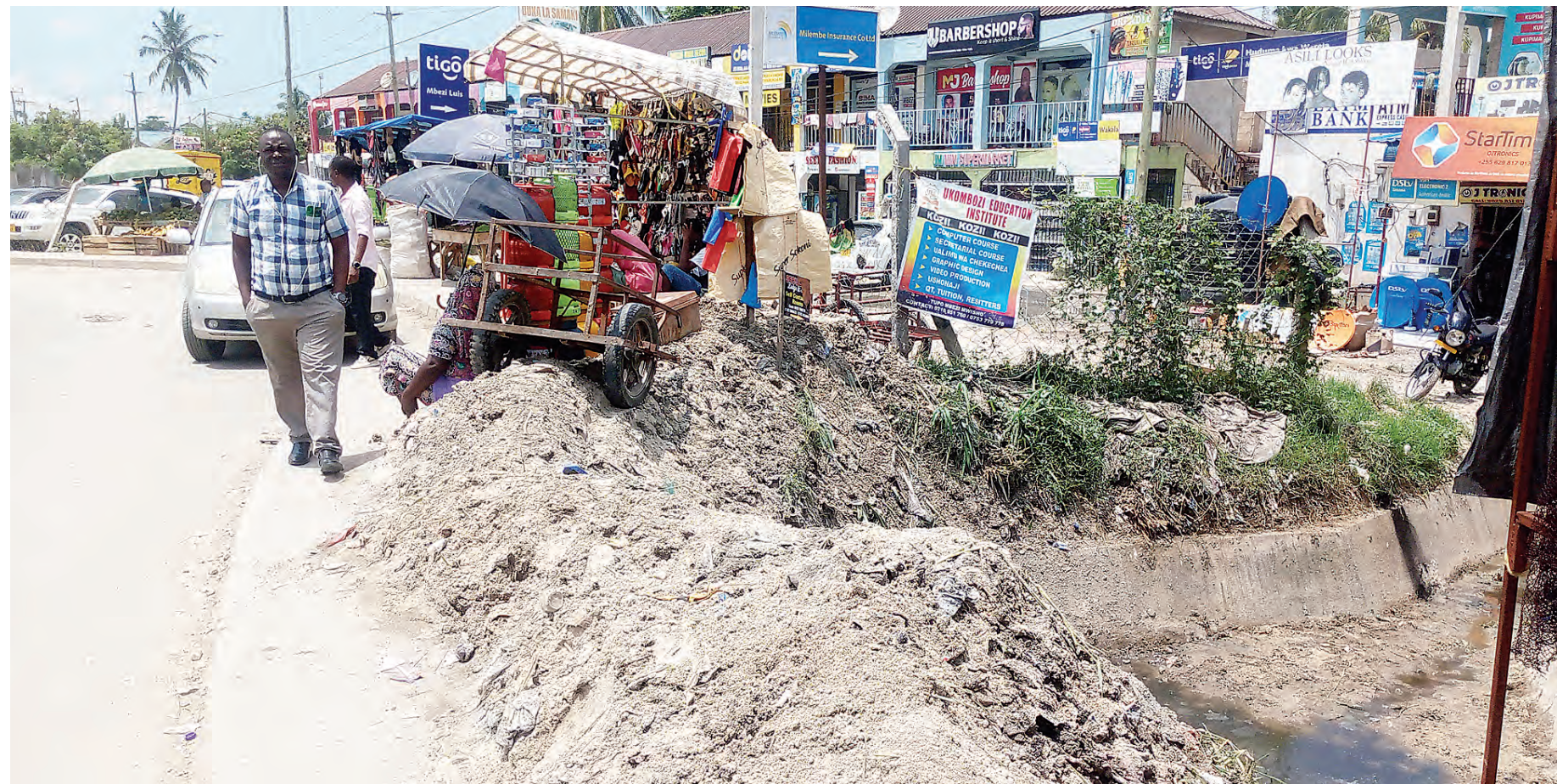
Sand cleared from a clogged roadside trench some days ago lies abandoned, as captured yesterday by our roving photographer at Mbezi Luis in Dar es Salaam's Ubungo Municipality. This could lead to a recurrence of the menace in case it rains again soon. Photo: Correspondent Sabato Kasika
