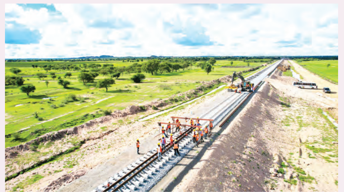
Workers are laying tracks at Seke Ididi, Kishapu District, Shinyanga Region for Lot 5 of the Standard Gauge Railway (SGR) from Isaka to Mwanza in February 2023. The project is undertaken by two Chinese construction companies, CCECC and CRCC. (Photo/CCECC)
