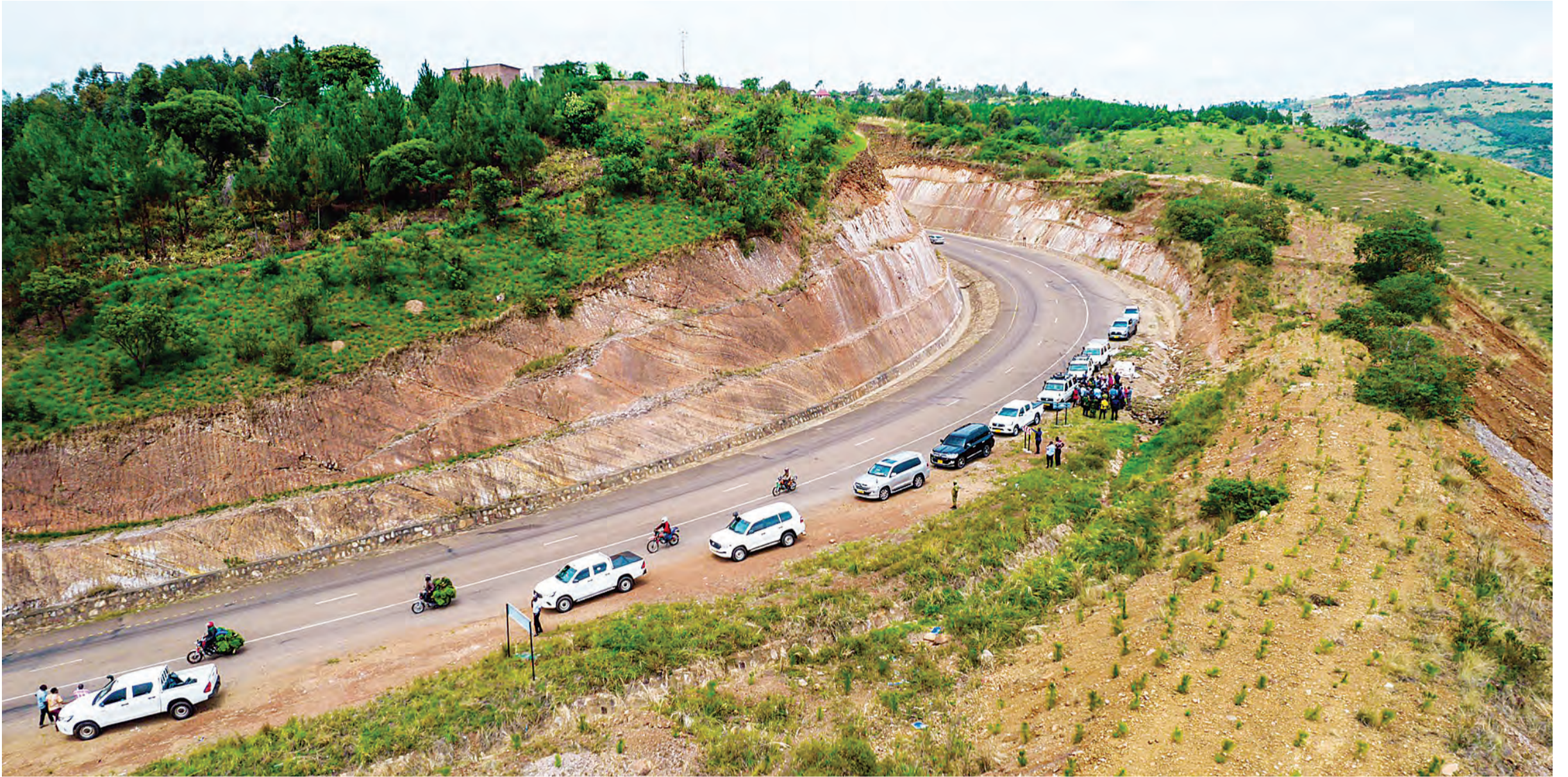
Residents of Kishoju Village in Kihanga Ward, Karagwe District, which this road passes through danced when it was first opened but that was cut short soon after vehicles started using it. Celebrations turned into funerals as fatal accidents occurred one after another. Photo/ Adonis Byemelwa
