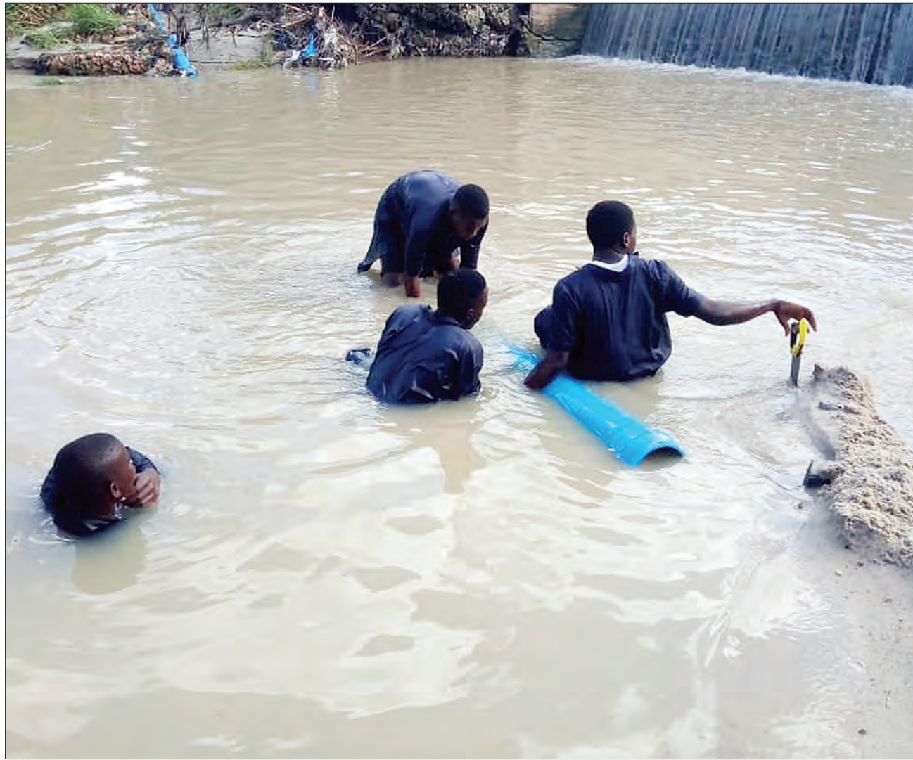
Dar es Salaam Water and Sanitation Authority (Dawasa) technicians have a challenging time working on a water pipe meant to run from Kimara to Tabata Kinyerezi via Bonyokwa, as captured yesterday. Photo: Guardian Correspondent
