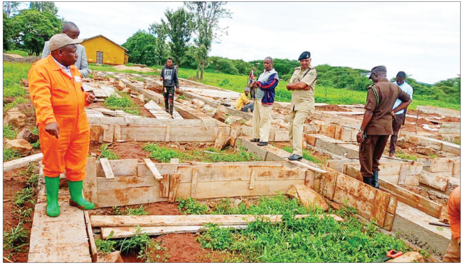
Mbulu District Commissioner in Manyara Region Chelestino Mofuga (L) accompanied by Defence and Security committee inspect construction of Maretadu secondary school's dormitory on Tuesday. Photo: Correspondent Gift Thadey
