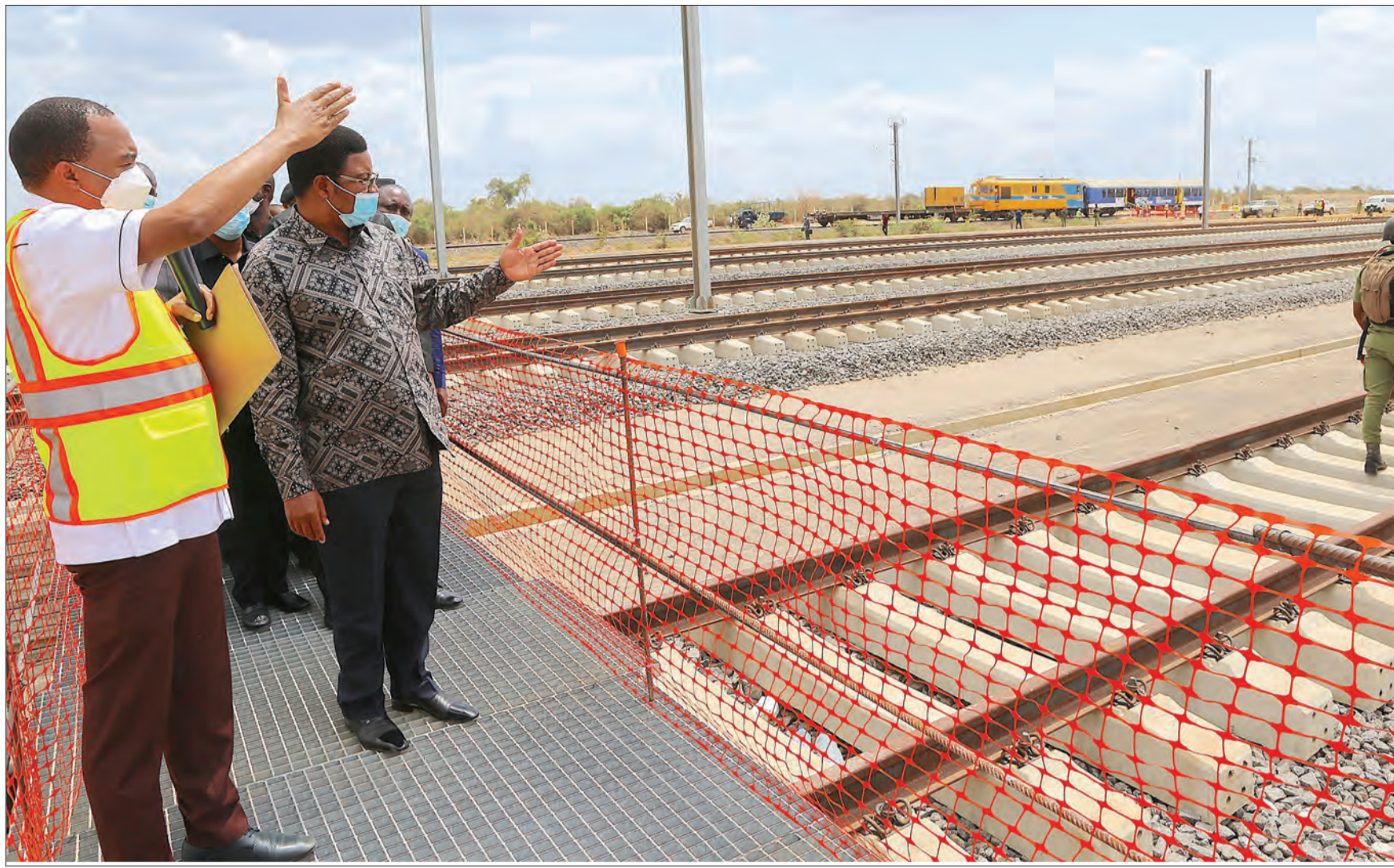
Tanzania Railways Corporation director general Masanja Kadogosa (L) briefs Prime Minister Kassim Majaliwa on progress in the construction of the Standard Gauge Railway workshop at the project's Kwala site in Coast region yesterday. Photo: PMO
