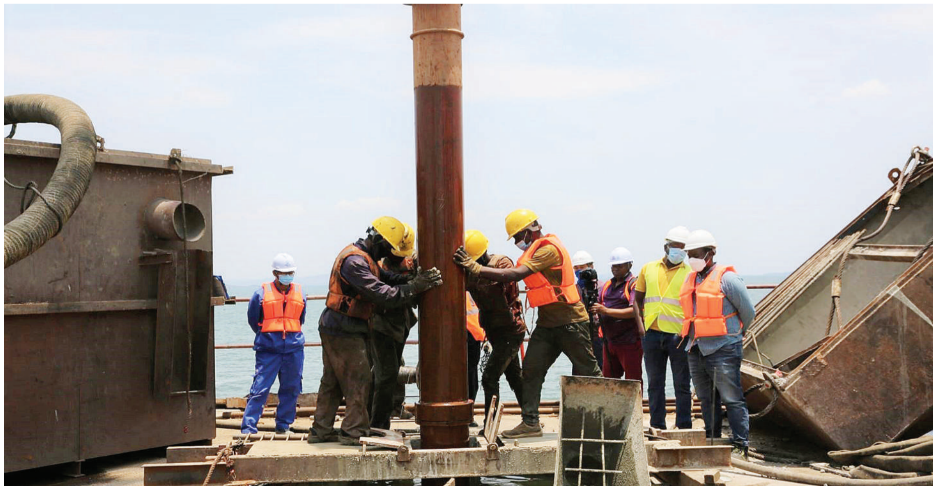
Installation of columns in progress yesterday at Mwanza Region's Kigongo-Busisi bridge, which is still under construction. The bridge is 3,200 meters long is scheduled for completion in February 2024. Photo: Guardian Correspondent
