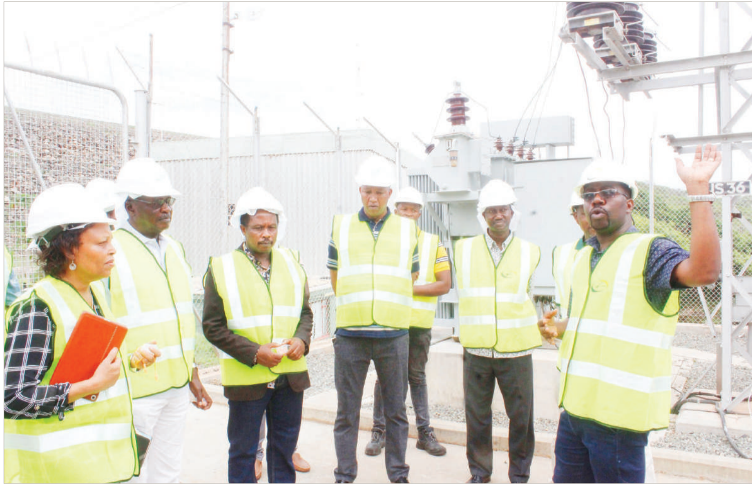
Nyumba ya Mungu dam electrical power acting manager Eng Edmund Seif (R) briefs Tanesco board members during a visit in Kilimanjaro Region recently. Photo: Correspondent Oscar Kasimiri
