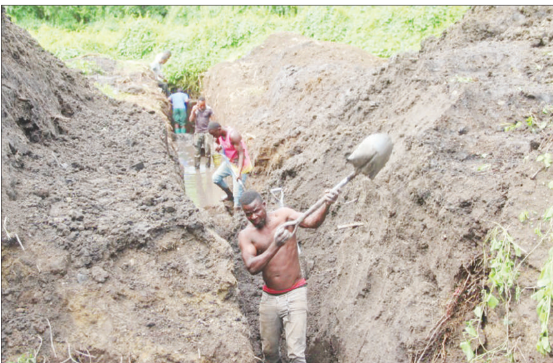
Mbeya Water Supply and Sanitation Authority workers dig a tunnel to supply water services for the residents of Nzovwe, Isyesye and Itezi. Photo: Correspondent Nebart Msokwa
