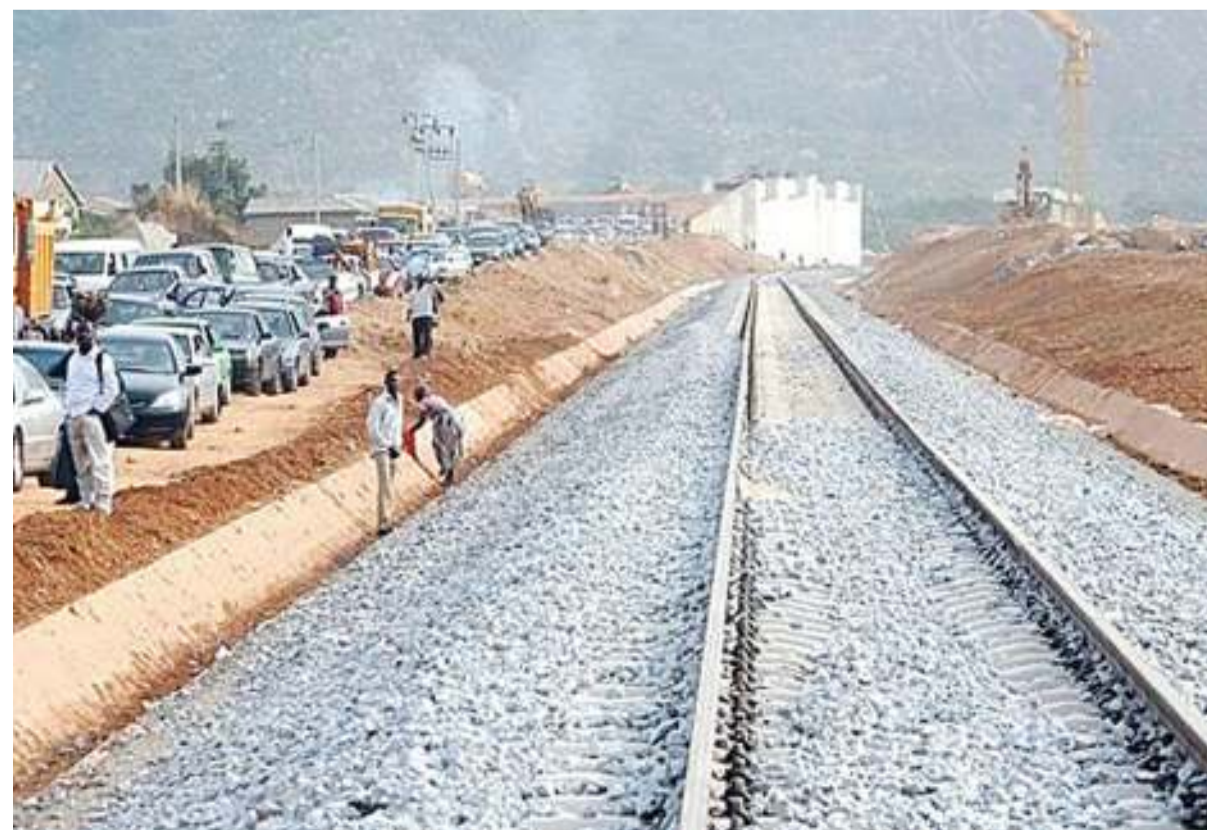
Construction work of the multi-trillion shillings Standard Gauge Railways going on in Dar es Salaam. File photo.
