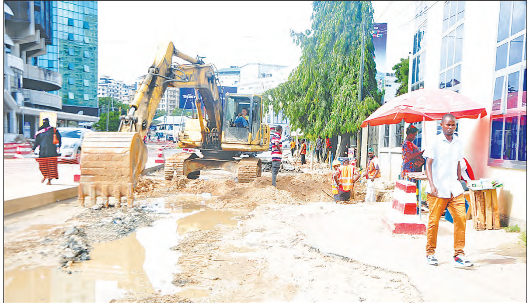
Despite the harsh conditions induced by a downpour, work continues yesterday in the implementation of Dar es Salaam's rapid bus transit (BRT) road project at the Bibi Titi Street/Azikiwe Street intersection. Photo: Correspondent Imani Nathaniel
