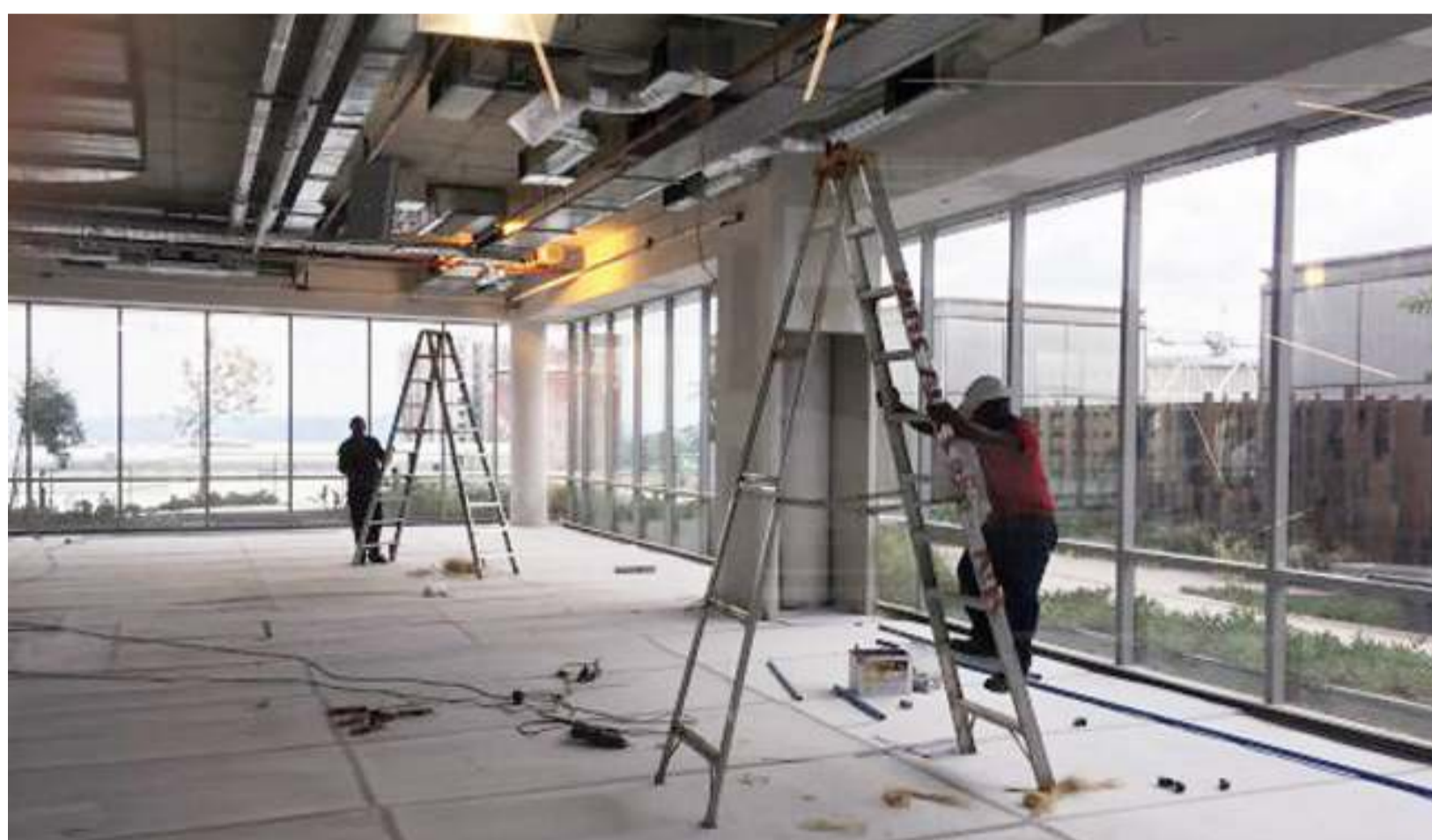
Tradesmen preparing the WeWork rental space at the R712m Rosebank Link building.
