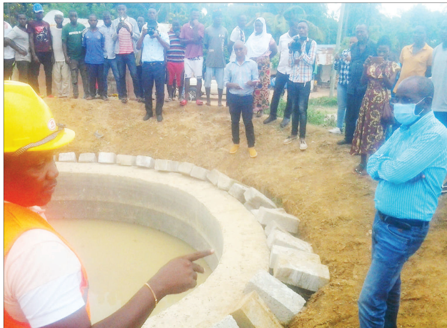
Juin Company Ltd contractor Innocent Bernard (L) briefs Water minister Prof Makame Mbarawa (R) yesterday on a tank the firm is building in partial implementation of a Muheza District water supply project. Photo: Correspondent Steven William
