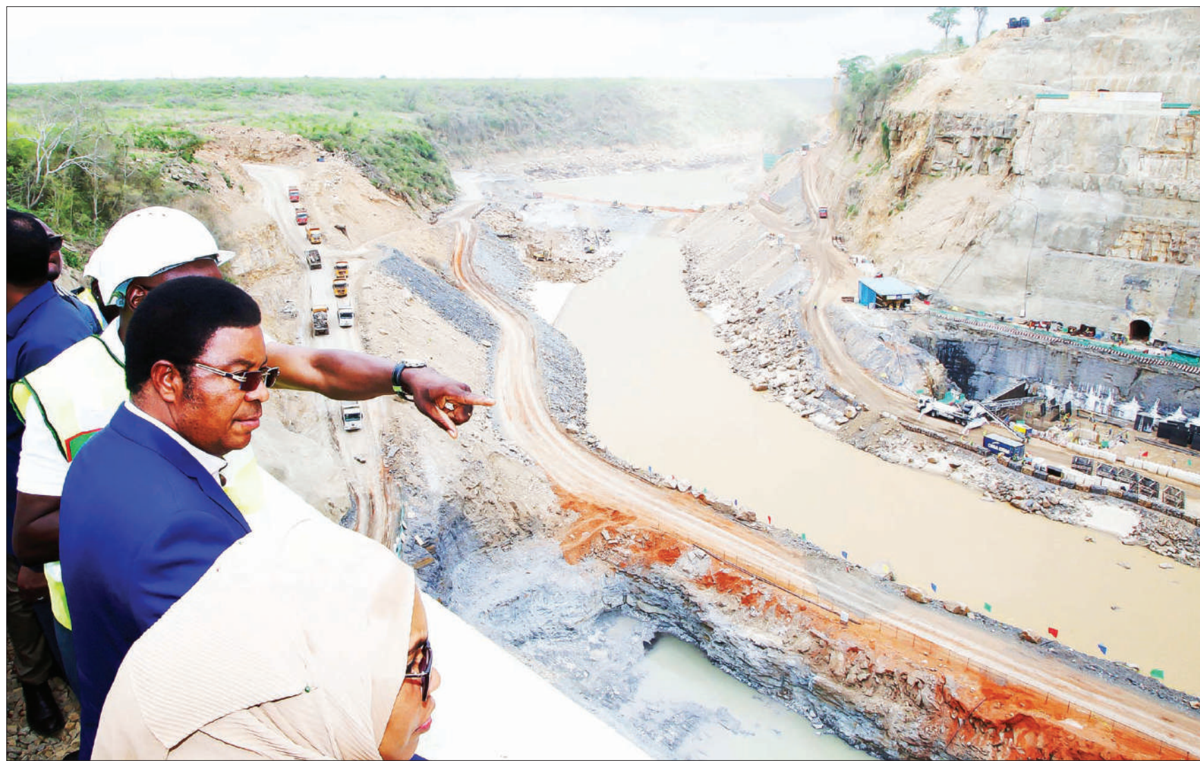
Prime Minister Kassim Majaliwa has a first-hand account at the Julius Nyerere Hydro Power Project site in Coast Region yesterday as he witnesses the diversion of the Rufiji River waters to a tunnel, the plan being to pave the way for the construction of the main hydropower dam. Photo: PMO
