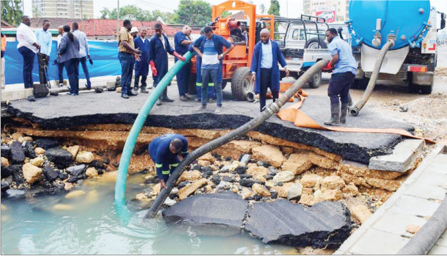
Dar es Salaam Water and Sanitation Authority technicians rehabilitate a major pipe near the city's Victoria commuter bus stand yesterday to end days of an acute shortage of water in the neighbourhood. Photo: Guardian Correspondent
