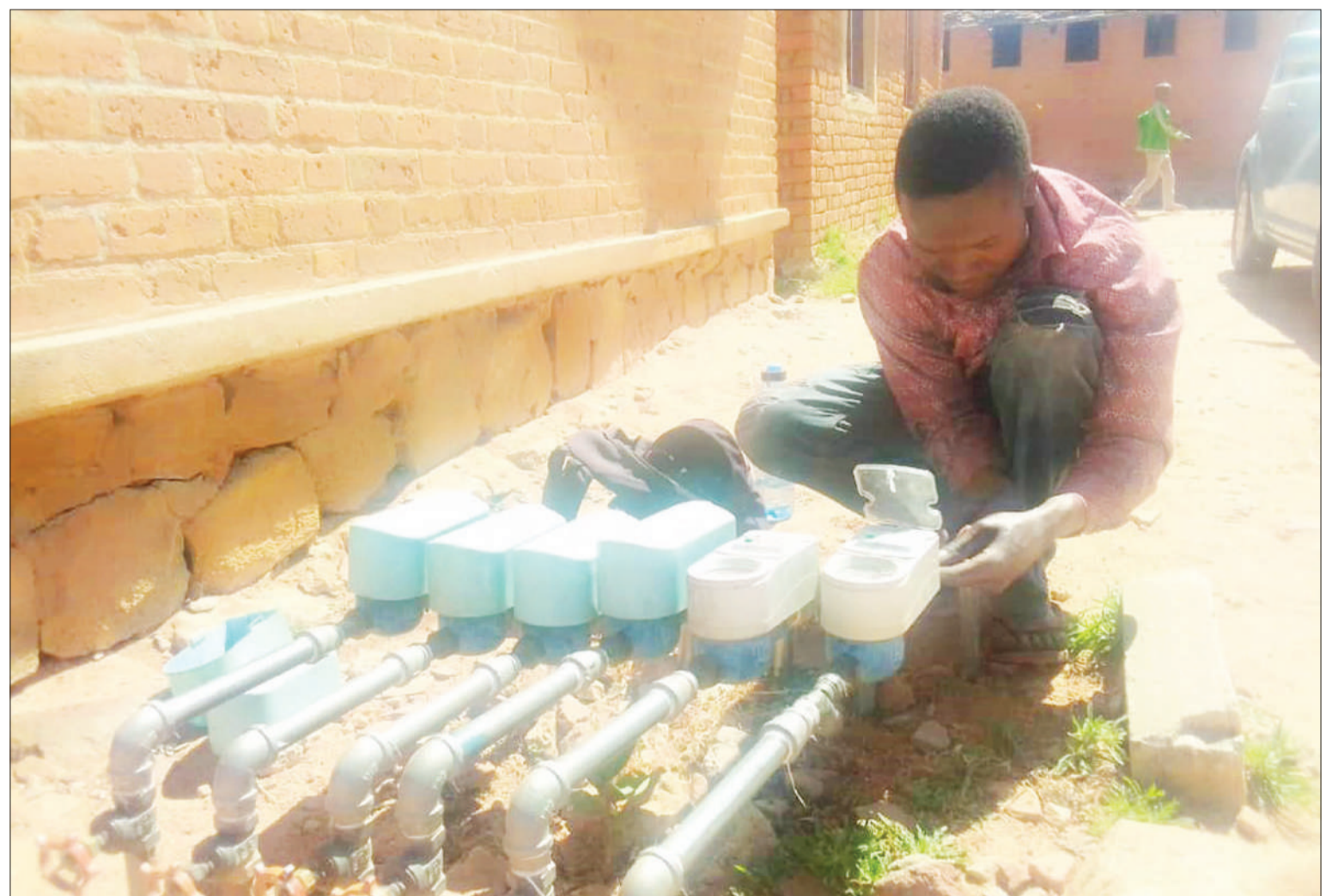
A technician with the Iringa Urban Water and Sanitation Authority installs prepaid meters for its customers, as found along Magereza Street in Iringa municipality yesterday. Photo: Correspondent Friday Simbaya
