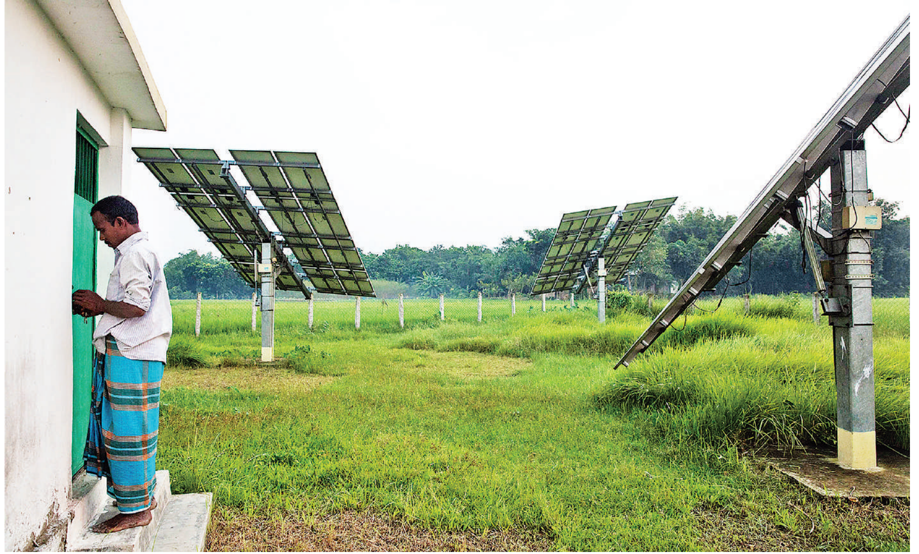
Solar irrigation for farmers and solar home systems for rural families installed by NGO Nusra in Bangladesh
