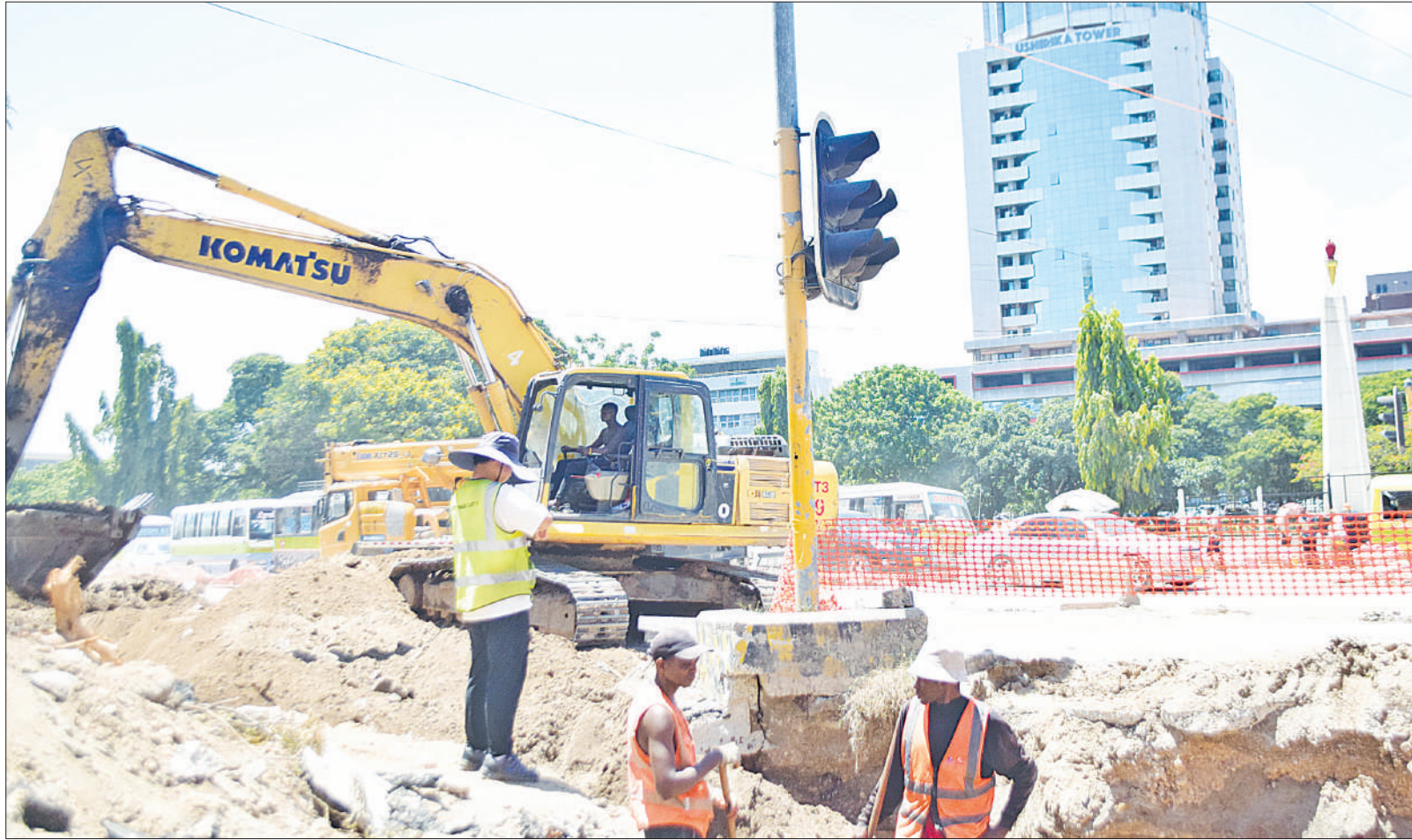
Work in progress at a Mnazi Mmoja section of Bibi Titi Street yesterday in implementation of Dar es Salaam's Bus Rapid Transit road project. Photo: Correspondent Jumanne Juma
