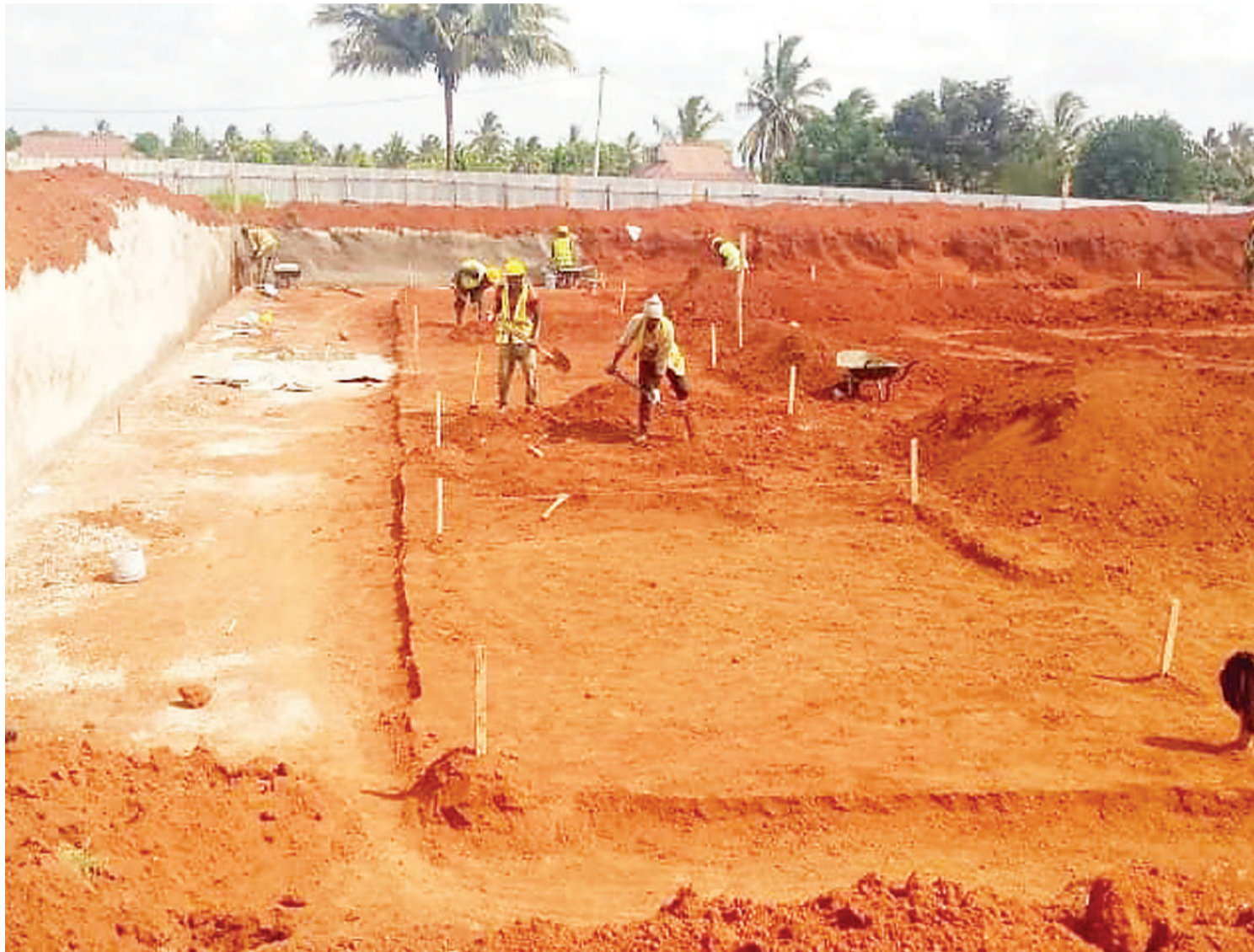
The Cedric and Hainan employees at work preparing a proper base for a water storage tank at Vikawe in Bagamoyo District, Coast Region. The project being under taken by Dar es Salaam Water and Sanitation Authority. Photo: Guardian Correspondent
