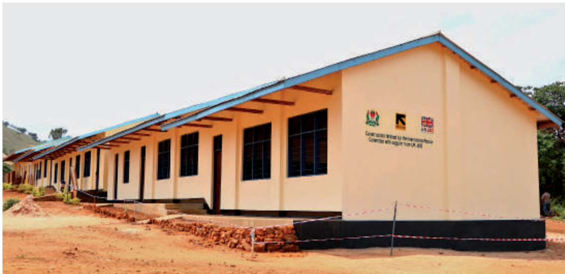
IRC worked with the local community finish construction of five new classrooms and two new office buildings at Mapinduzi Primary School in Kibondo DC
