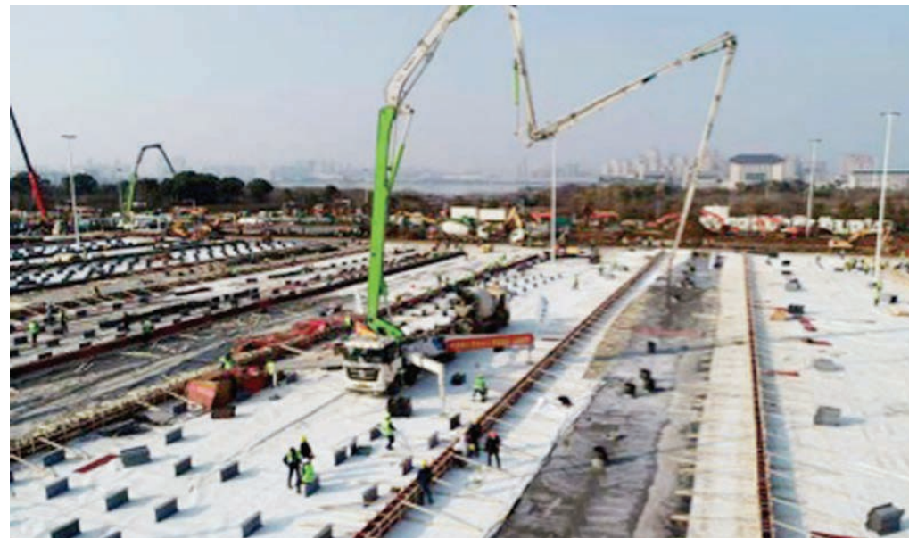
Photo shows the construction site of Huoshenshan Hospital in Wuhan, capital of central China's Hubei Province. (Photo by Wang Wei/People's Daily)
