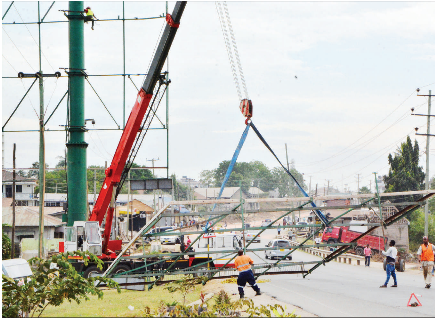
Advertising agents pull down a billboard yesterday to pave the way for the expansion of Dar es Salaam's Shekilango Road. Photo: Correspondent Miraji Msala
