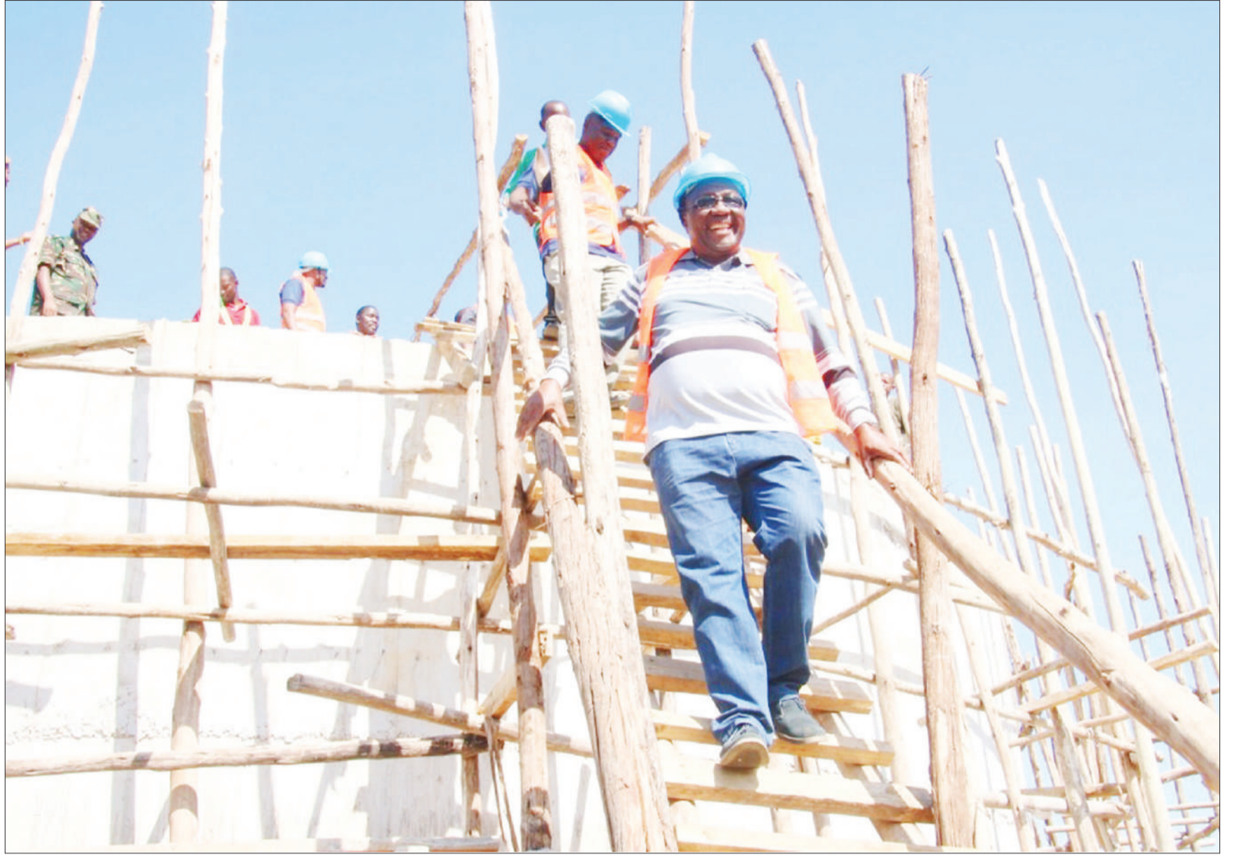
Kahama district commissioner Anamringi Macha descends from the top of a water tank being built by the Shinyanga Urban Water and Sanitation Authority in implementation of a project meant to supply Shinyanga municipality and its environs with water from Lake Victoria at a cost of 2.4bn/- Photo: Correspondent Shaban Njia
