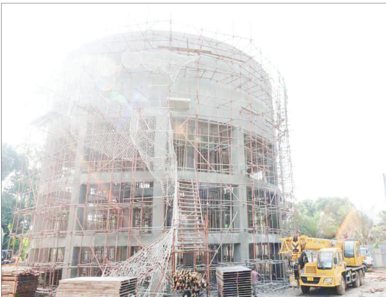
This 1.5-million-litre water tank is undergoing construction as part of a Mkuranga-Vikindu project in Coast Region. It is meant to supply water through 63.5 kilometres of pipes and a booster station, benefiting some 25,000 people. The scene was captured at the weekend. Photo: Guardian Correspondent
