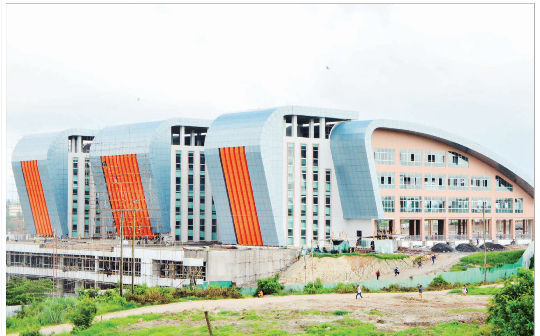
SLOWLY BUT SURELY TAKING SHAPE: This is a scene from the modern long-distance bus terminal undergoing construction at Mbezi Mwisho in Ubungo District, Dar es Salaam, as captured yesterday. The facility is expected to have 'trial runs' any of these days, according to authoritative sources. Photo: Correspondent Miraji Msala
