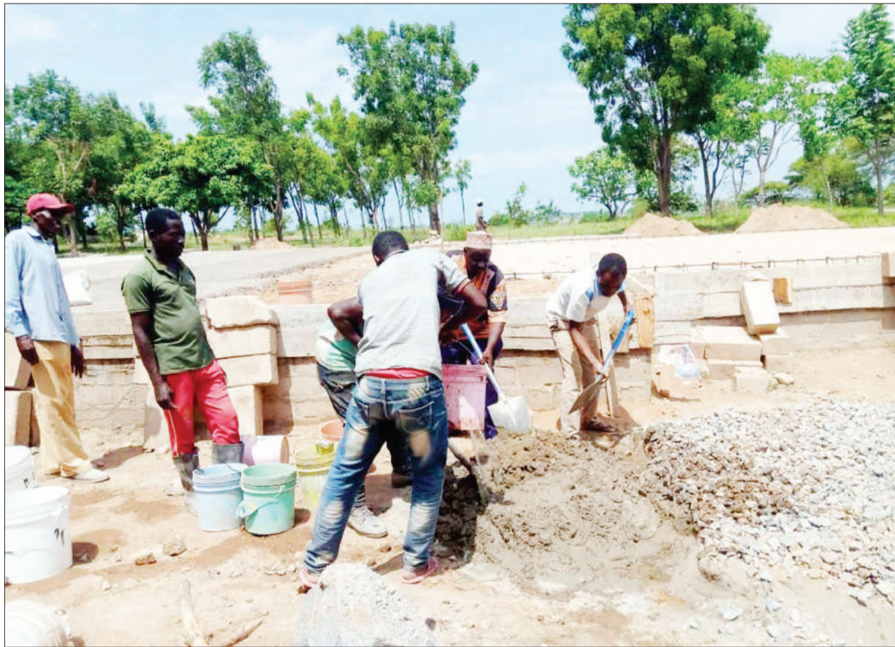
The construction of the administration block for Kiriba Secondary School in Musoma Rural constituency has begun, as found yesterday, with headmaster Paul Mtani saying the government has released 50m/- to help expedite the work. Photo: Guardian Correspondent
