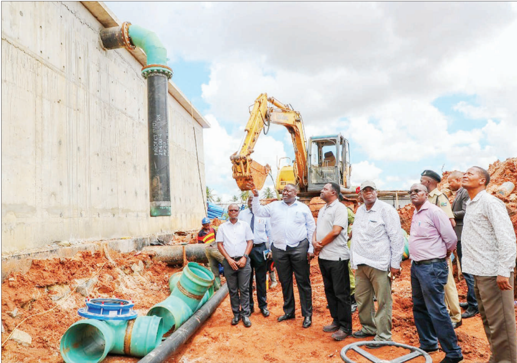
Dar es Salaam Water Supply and Sanitation Authority (Dawasa) CEO Cyprian Luhemeja (2nd-L, foreground) briefs Dar es Salaam regional commissioner Abubakari Kunenge (to his left) on the implementation of the Kisarawe-Pugu-Gongo la Mboto water project. The RC made an inspection tour of the project yesterday. The Dawasa CEO promised that all residents of Pugu and Chanika would have access to safe and clean water by the end of next month. Photo: Guardian Correspondent
