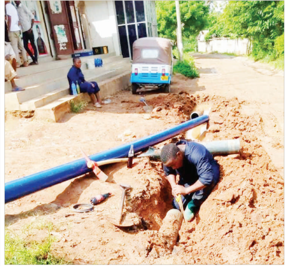
A Dar es Salaam Water and Sanitation Authority (Dawasa) technician moves to repair a leaking water pipe at Mbezi Msakuzi in Ubungu District yesterday. Photo: Guardian Correspondent
