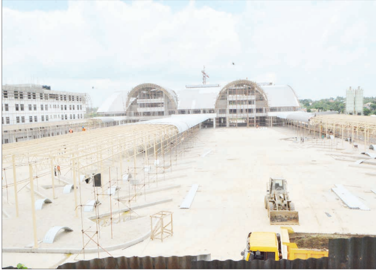
Workers putting final touches on new Dar es Salaam International Bus Stand at Mbezi Mwisho in Ubungo District as captured yesterday. Photo: Correspondent Moraji Msala
