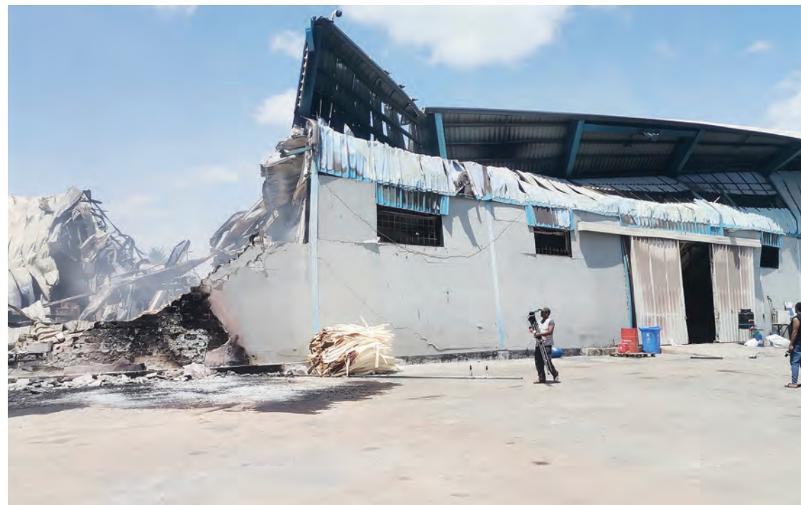
FACTORY GUTTED BY FIRE: This is about all that was left at the Mikocheni Light Industrial site in Dar es Salaam of what was until dawn yesterday GSM foam mattress factory after it was hit by a raging fire in circumstances yet to be conclusively established. Photo: Jennifer Gilla
