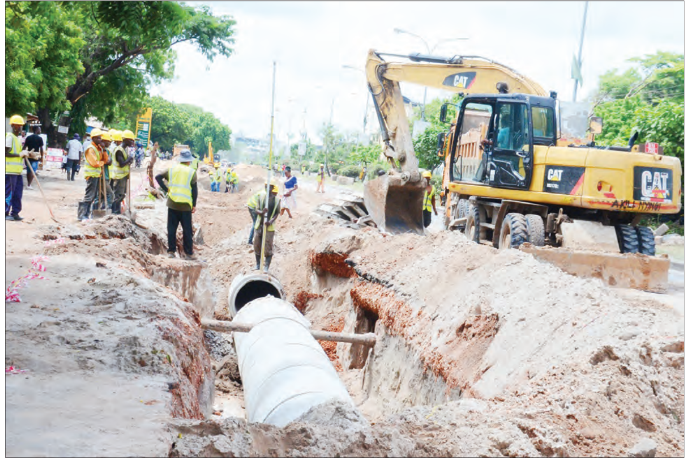
Construction of a sewage system in progress yesterday as part of the implementation of the Ilala section of the second phase of Dar es Salaam's rapid transit bus project. Photo: Correspondent Jumanne Juma
