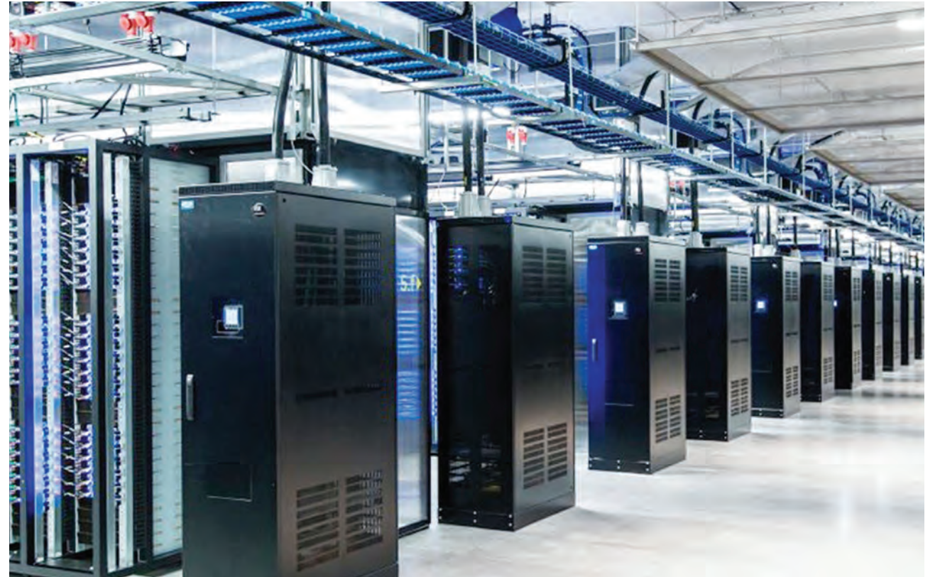
A data centre
