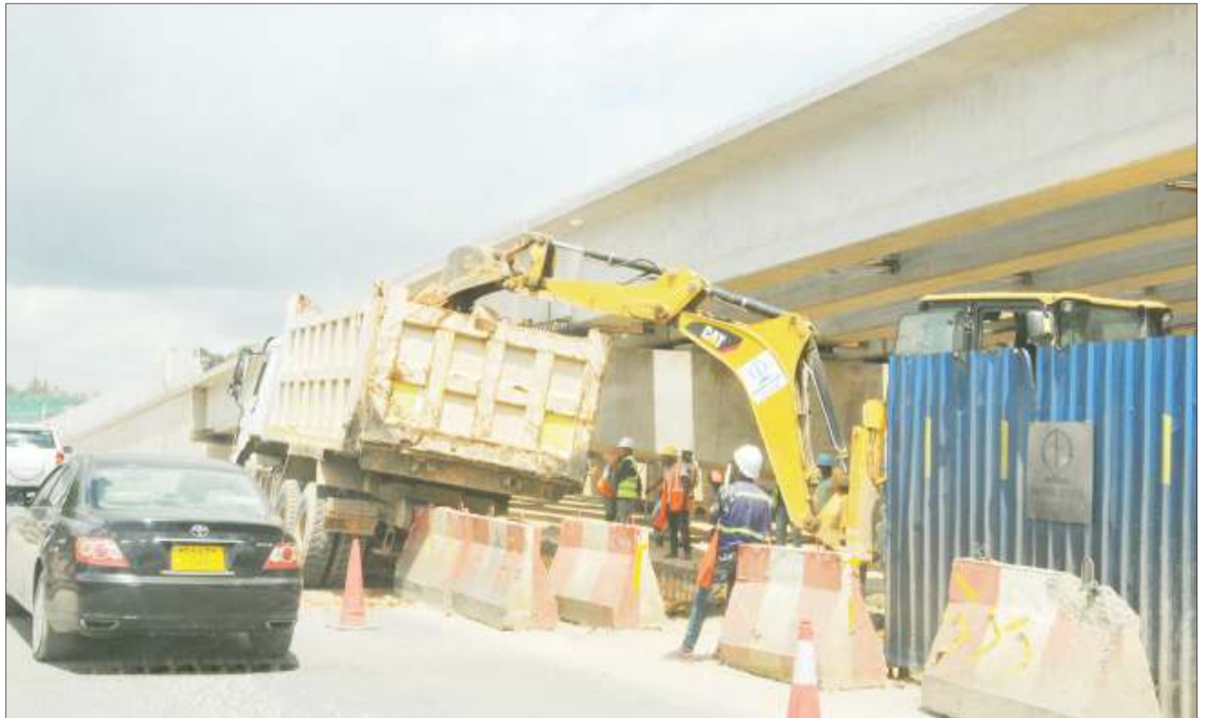
A section of Dar es Salaam's Ubungo Interchange, which is still undergoing construction at the Morogoro Road/Mandela Road/Sam Nujoma Road intersection, as captured on Monday. Photo: John Badi
