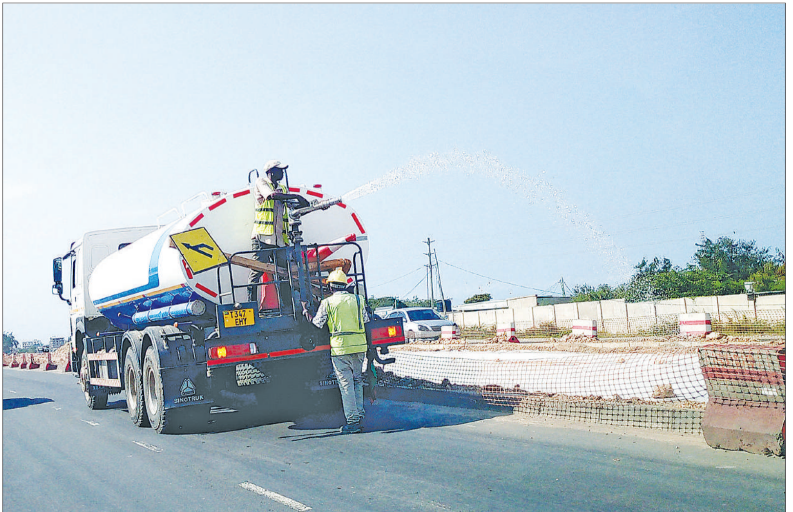
This is part of evidence of the ongoing implementation of Dar es Salaam’s rapid transit bus infrastructure project, as found yesterday along the Lugalo stretch of Bagamoyo Road. Photo: Correspondent Sabato Kasika
