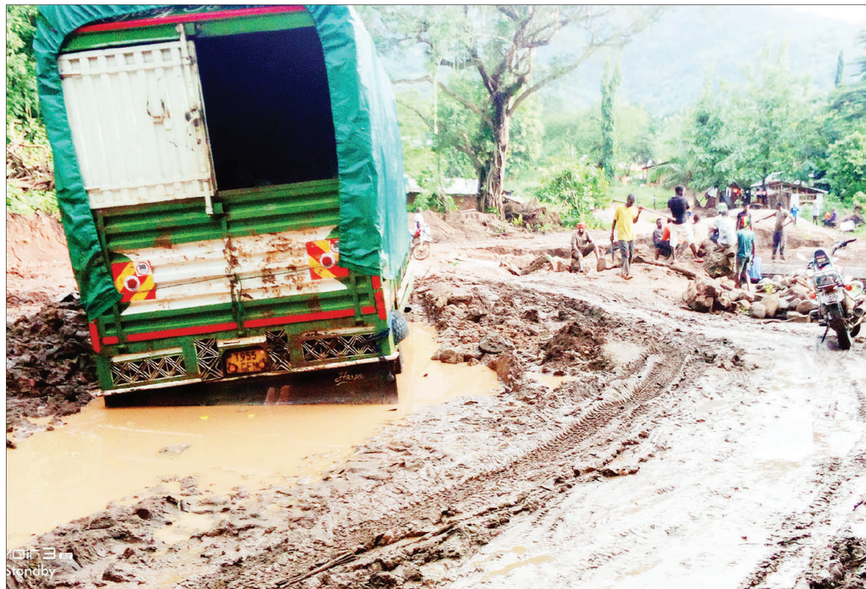
A truck lies stuck in the mud yesterday at a spot between Mashewa and Bombani villages in Muheza District, as Tanzania National Roads Agency (Tanroads) workers move to repair a bridge damaged by recent rains. This has made farmers in the area face serious problems transporting their crops to Muheza market. Photo: Correspondent Steven William
