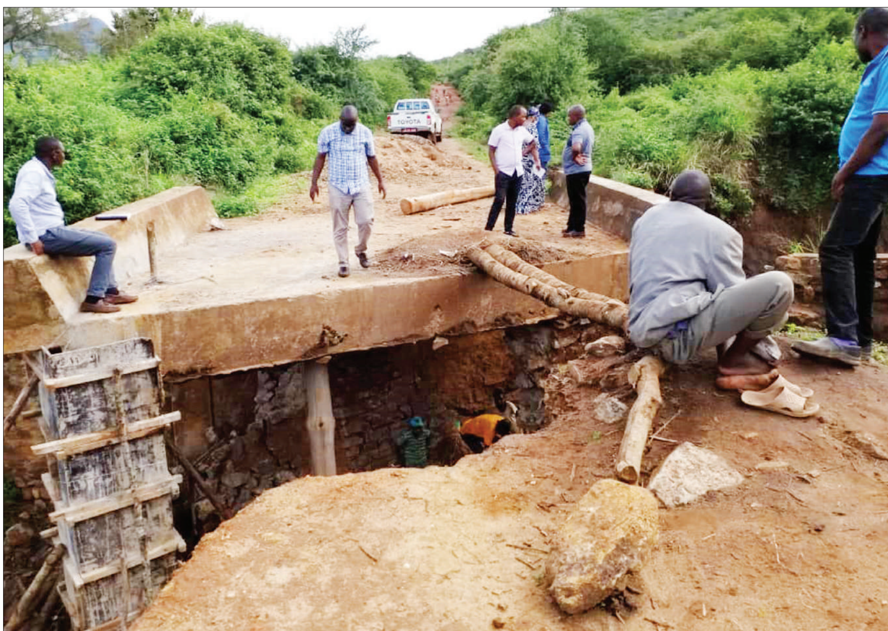
Rehabilitation of a bridge connecting Kisiwani and Msindo in Same District in progress, as found yesterday. It was damaged by recent rains. Photo: Godfrey Mushi
