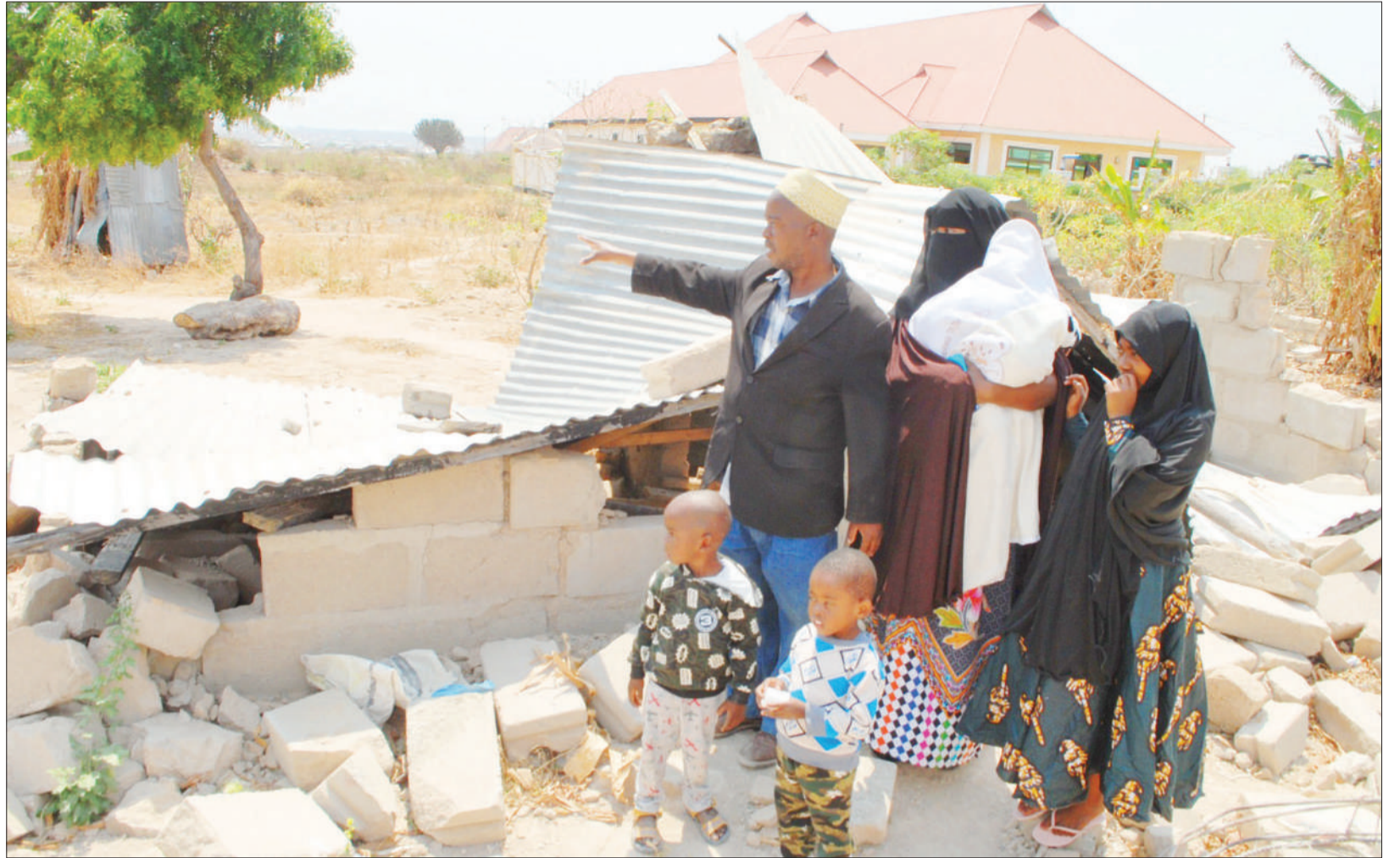
Said Salum of Ndachi B Centre Block D in Dodoma looks on forlornly yesterday with members of his family next to what used to be his house in the national capital before it was pulled down, reportedly on instructions from "the relevant authorities". Photo: Correspondent Peter Mkwavila
