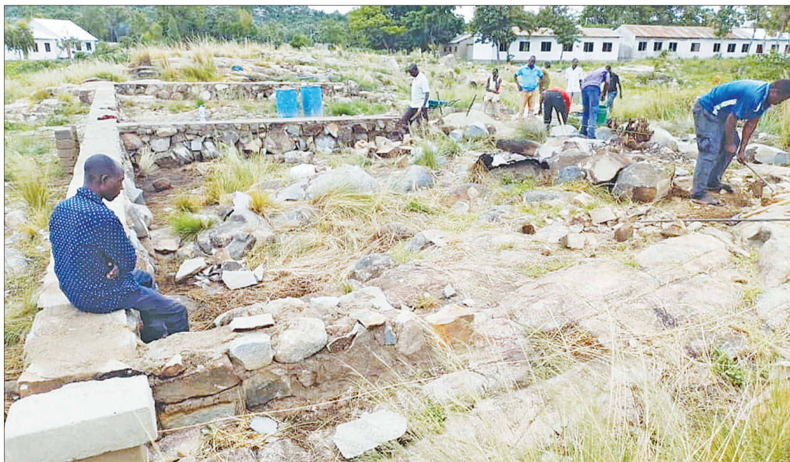
Construction of a classroom building at newly established Rukuba Island Secondary School in Musoma Rural constituency at initial stage, as captured yesterday. Photo: Guardian Correspondent
