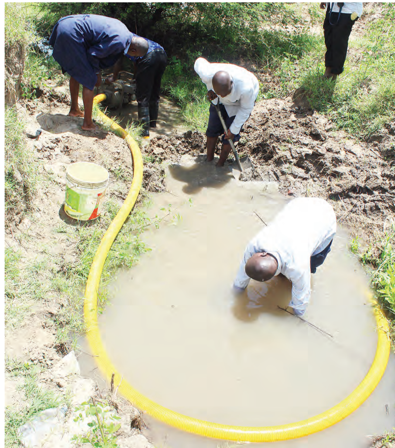
Shinyanga Urban Water Supply and Sanitation technicians fight to remove water to pave the way for the fixing of a leaking water pipe at Masekelo near River Kidalu yesterday. Photo: Correspondent Marco Maduhu
